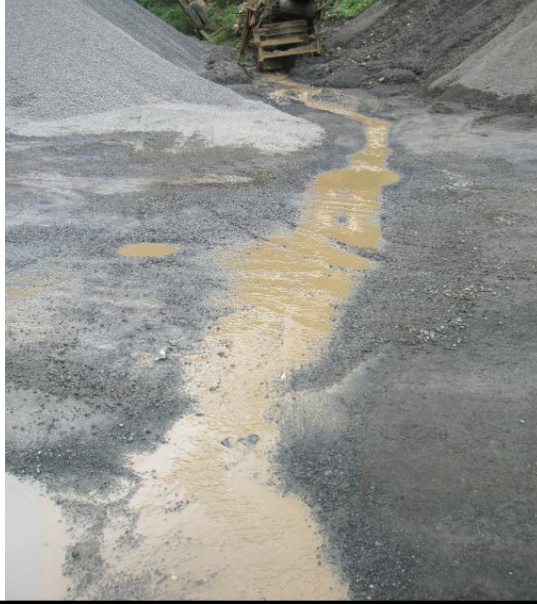
Photo 5 – View looking back uphill at the seepage after it has traveled down the primary driveway, squeezed between the gravel stockpiles and back across the driveway
