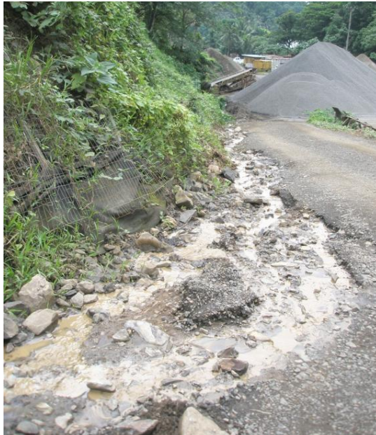
Photo 4 – Groundwater seep from excavated area collects and is conveyed down the primary driveway to the site
