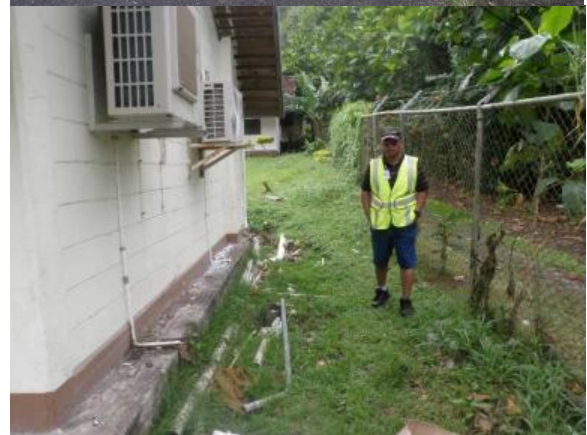
Figure 7B. Proposed location for small bioretention between building rows. Exposed sanitary sewer line and stormwater converging in one location at the outlet of Area B.
