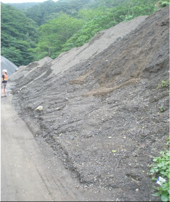
Photo 13 – Stockpile instability immediately adjacent to main driveway
