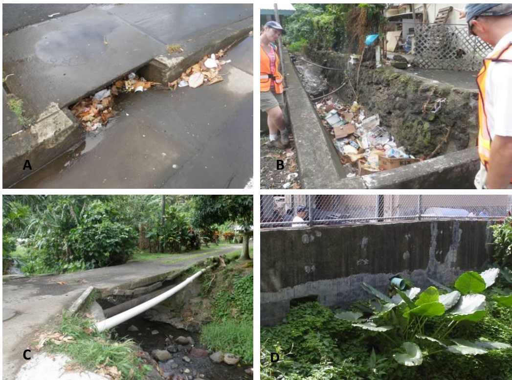
Figure 5. Drainage infrastructure that requires both routine and long-term maintenance includes A) catchbasins, B) culverts, C) bridges, and D) outfall pipes.
