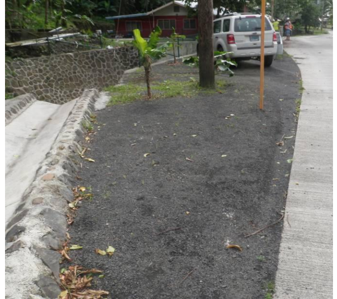
Figure 2B. Existing concrete swale discharges directly to stream. There is additional evidence of flow paths eroding gravel parking pad.
