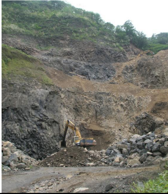
Photo 3 – View looking up at excavator operating at toe of rock face. Switch back haul road (3 turns) is seen winding up the hill side in background .
