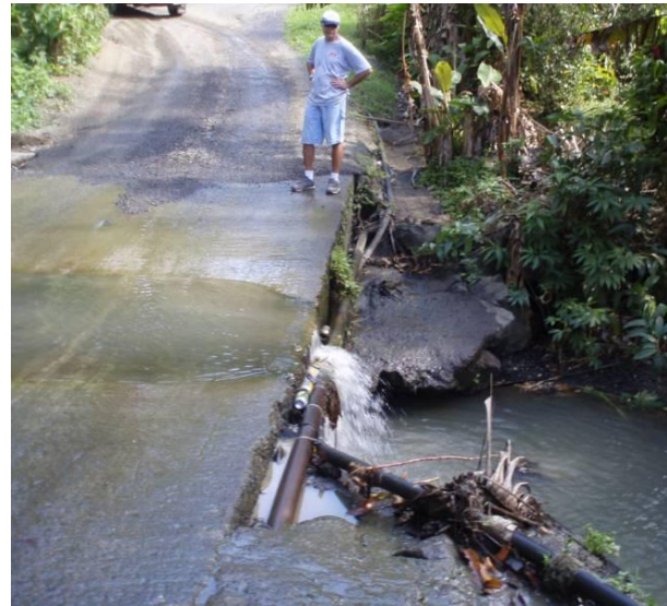
Figure 15A. Stream baseflow pouring across the road surface.
