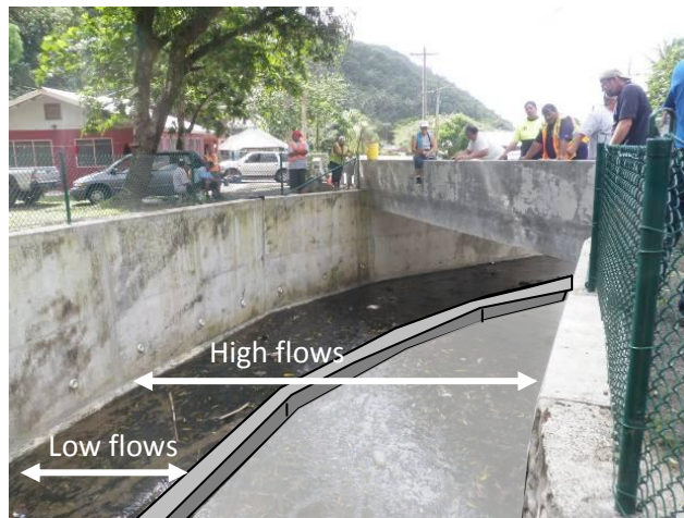
Figure 1A. Installation of 6-inch concrete berm to concentrate low flows to one side of channel. Flows higher than separator wall can spread across entire channel width.
