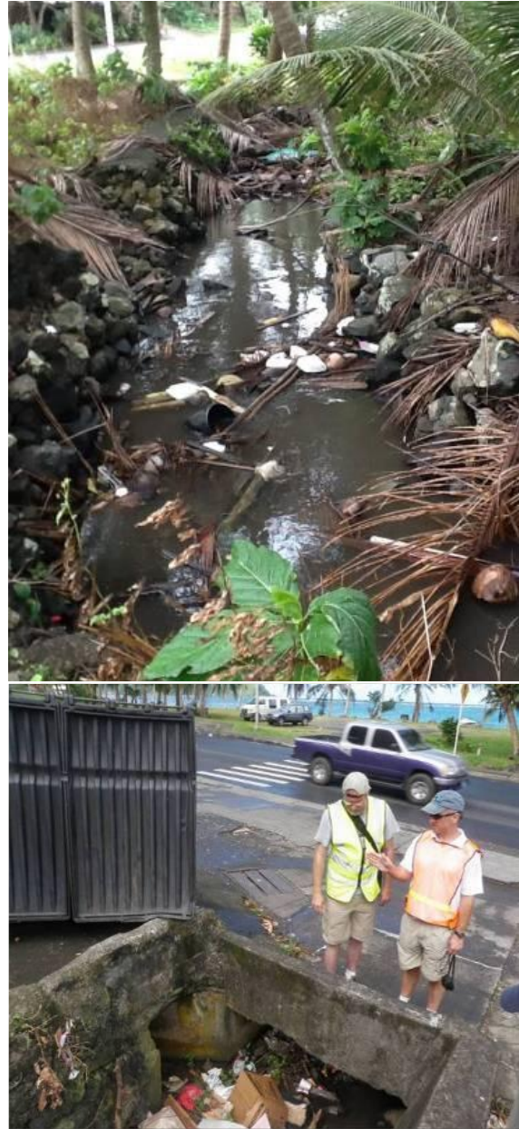
Figure 6B. Impacted stream section through park (top photo) and trash collected at upstream end of culvert (bottom).
