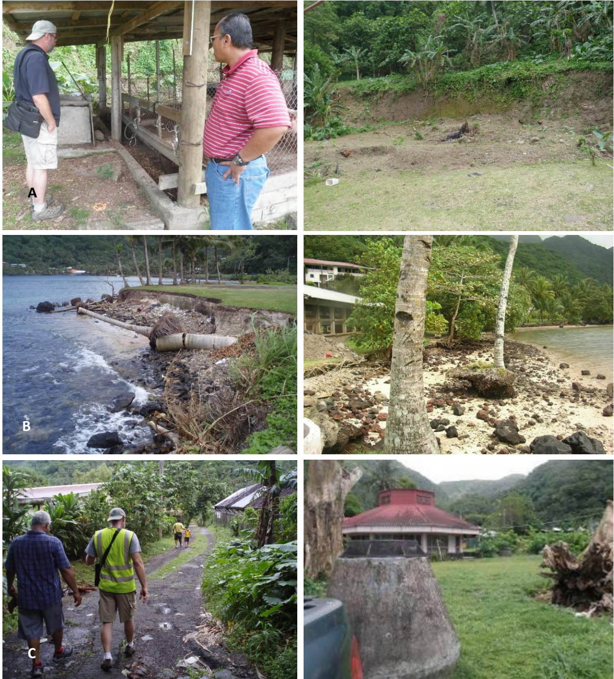
Figure 4. Structural projects not further described in Appendix A are: A) Site ID #13 completion of a dry compost piggery expansion project (small upgrade and cut slope at new location shown here); B) ID #9 and #11 shoreline stabilization at Matafao Elementary School and Faga’alu Park shown here, respectively; and C) ID #8 sewer extension and road improvement project for residential area above the Dept. of Health.
