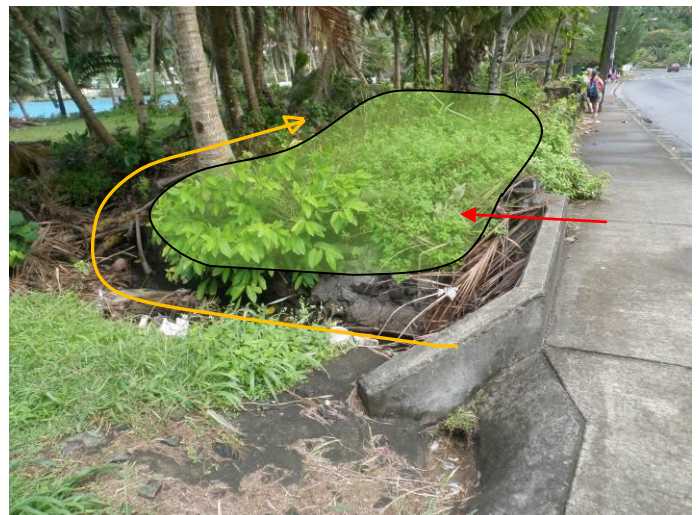
Figure 6A: Gravel wetland area, inflow diversion from new pipe across Hwy 001 shown in red arrow, bypass of flow from existing channel in orange.
