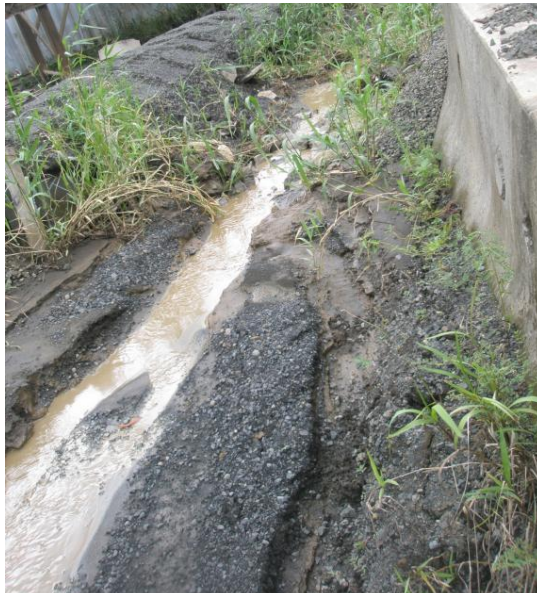
Photo 6 – Groundwater seepage (and runoff during rainfall events) eventually leaves the site through a small channel between jersey barrier and gravel berm, and an undersized sediment trap.
