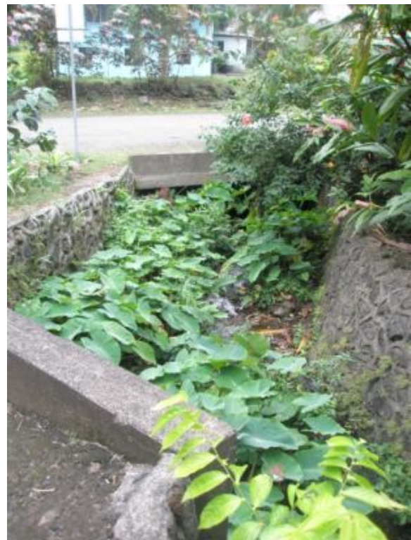
Figure 3B – Looking downstream at rectangular culvert under main road (outlet of existing culverts hidden by vegetation – no picture available).
