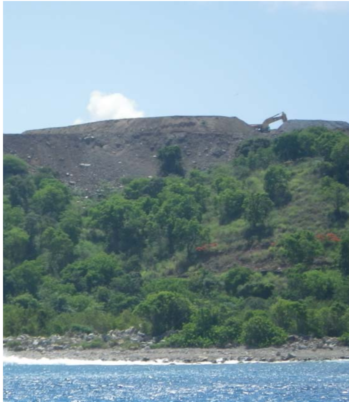
Figure 12. Excavation activity on Little St. James Island, a possible source of terrigenous sediments found in the sediment traps at this site.
