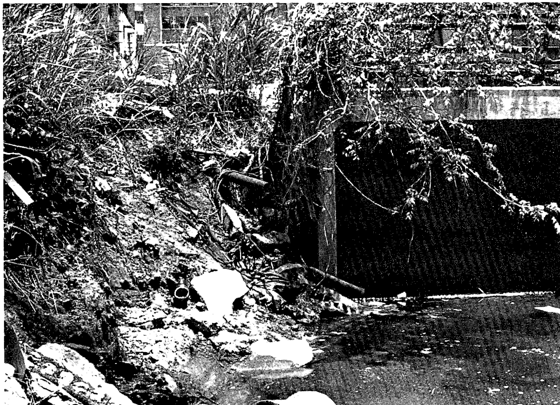
The almost-familiar sight of streambank erosion, illicit discharge pipes, and litter adding to a polluted urban stream in Raleigh, North Carolina.
