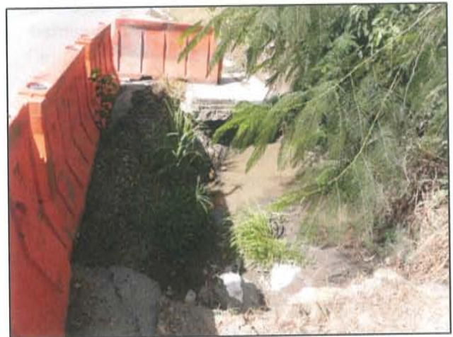
TR-40 showing hazardous conditions below Mariendahl neighborhood.
