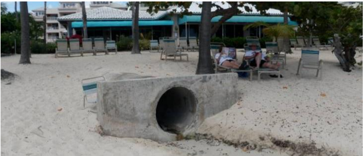
Discharge pipes visible on the beach drain parking lots, roads, and other developed areas in the watershed. In most cases throughout STEER, this runoff is not cleaned prior to discharge.
