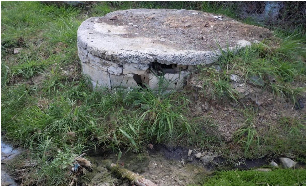
Deteriorating on-site sewage systems and evidence of recent wastewater discharges to guts were observed at multiple locations in the watershed.
