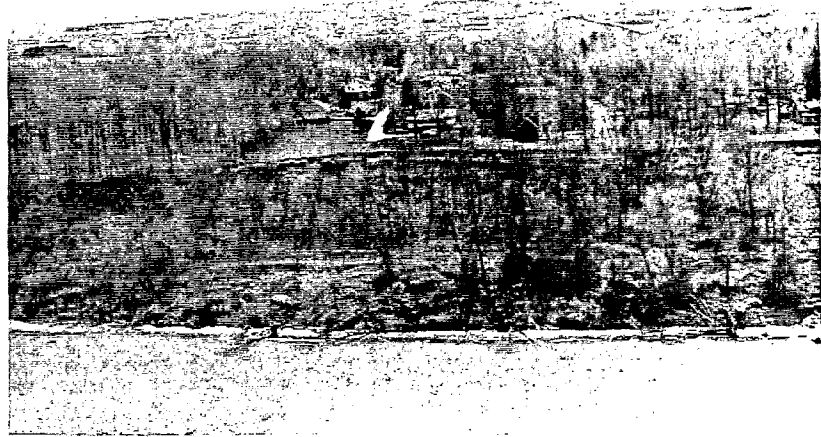
Above: An area of slumping due probably to increased infiltration of ground water because to vegetation cover at crest
