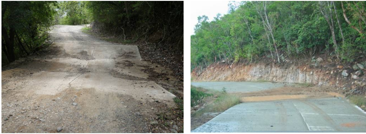
Figure 30. Dip constructed on an unpaved road (left) and one used on a paved road (right) in Coral Bay as an alternative to convey flow from both the road surface and from the inslope ditch to outslope.
