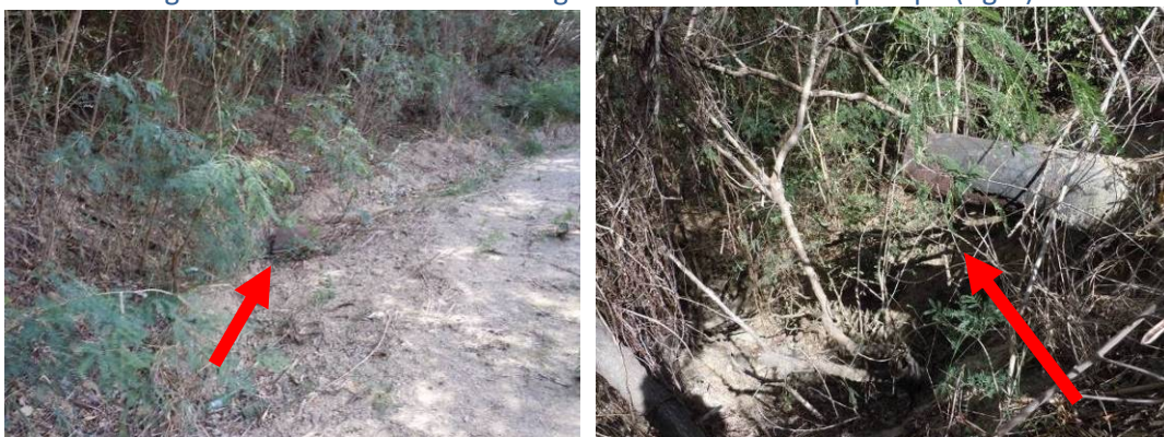
Figure 17. The upgradient end of the culvert is clogged with sediment, severely reducing its capacity (left), and the downgradient end has created a large scour hole on a steep slope (right).
