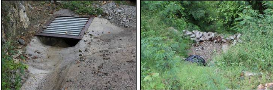
Figure 34. A drop inlet and culvert installed as a road improvement project in Coral Bay (Source CBCC).
