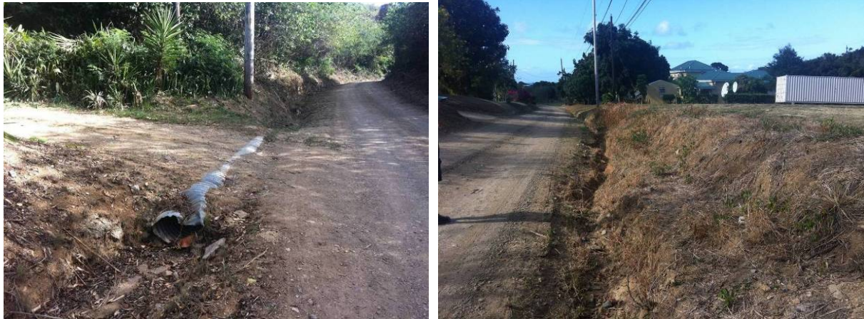
Figure 13. Damaged driveway culvert (left) and the eroding ditch serving as the gut (right).
