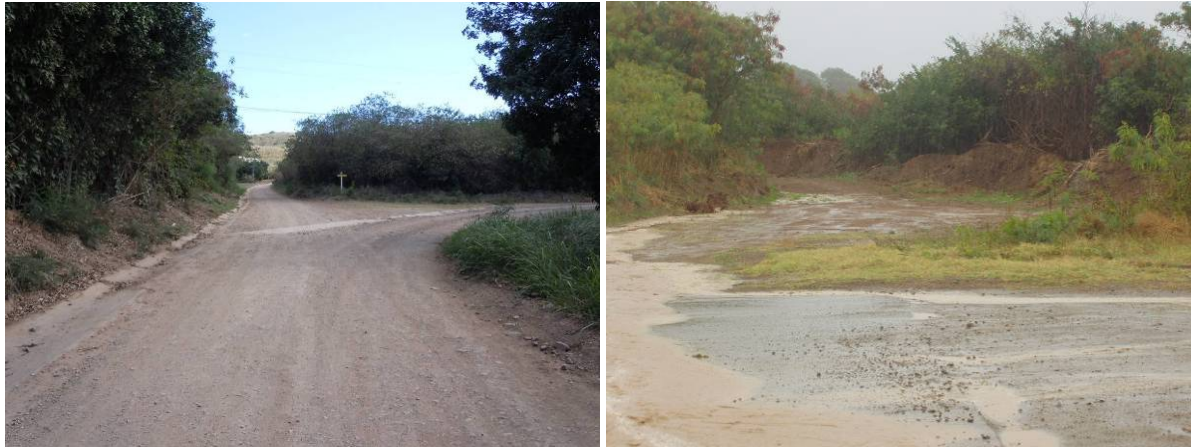
Figure 14. Shallow, paved swales at the downgradient end of Segment 4 (left), and a manmade drainage path created to help runoff reach the main gut – note piles of sediment exposed to runoff (right).
