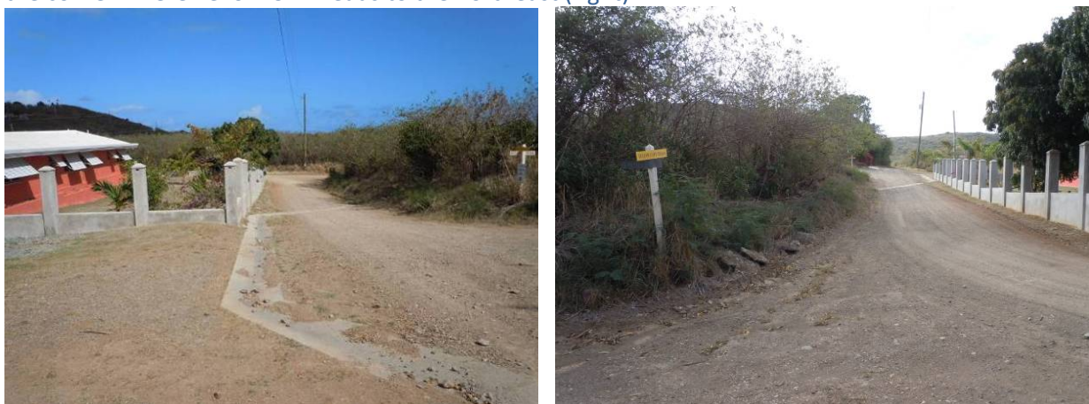
Figure 21. Shallow, paved swales at intersection with Hibiscus Circle (left), and the eroded ditch along the corner where Yellow Cliff heads to the northeast (right).
