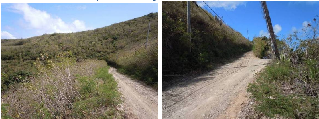
Figure 16. Yellow Cliff Trail is steep with an eroding ditch on the inslope.
