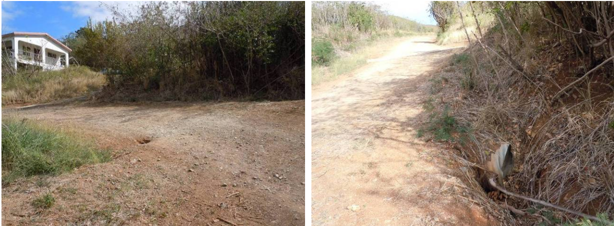
Figure 19. Clogged and damaged 24-inch corrugated metal culvert that carries runoff from the south portion of Hibiscus Circle across to the gut.
