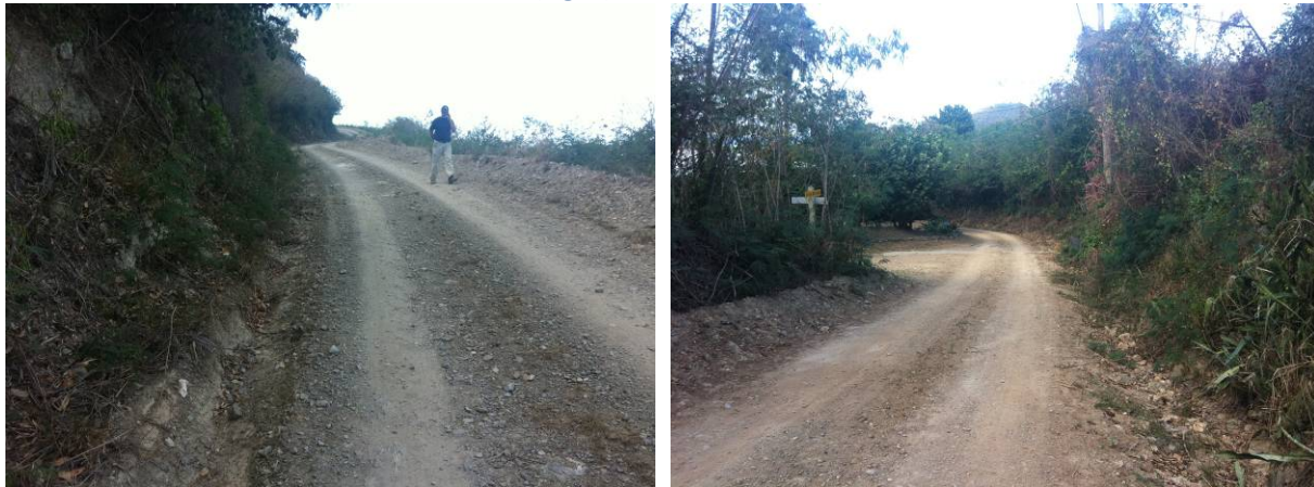
Figure 12. In some areas, the road has been graded down to the bedrock (left) with an eroding ditch on one side and earthen berm on the other (right).
