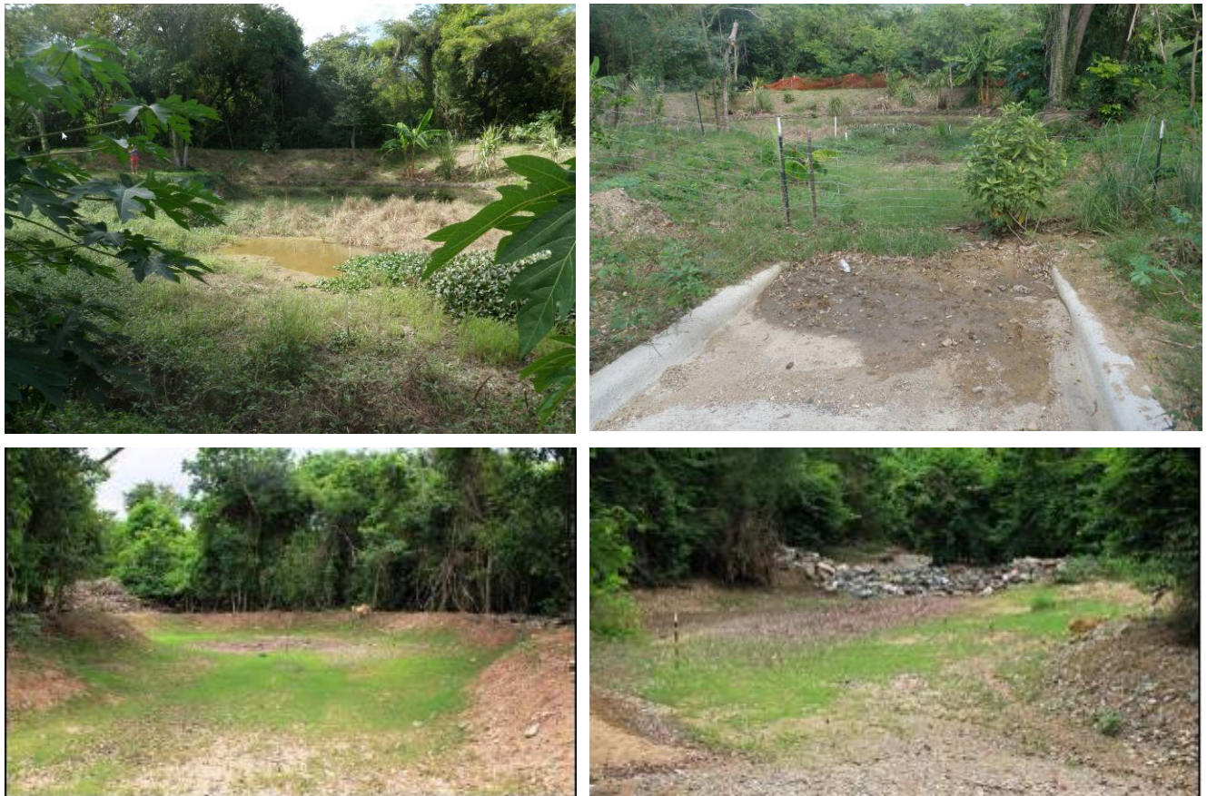
Figure 39. Wet vegetated pond retrofit in Coral Bay that manages runoff from Kingshill Road. Sediment accumulation is evident in the paved flume from the road leading to the practice (Top). The facility is being monitored to determine how much sediment is collected. Infiltration/sediment basin constructed in Carolina drainage in Coral Bay (Bottom, photos courtesy of CBCC).
