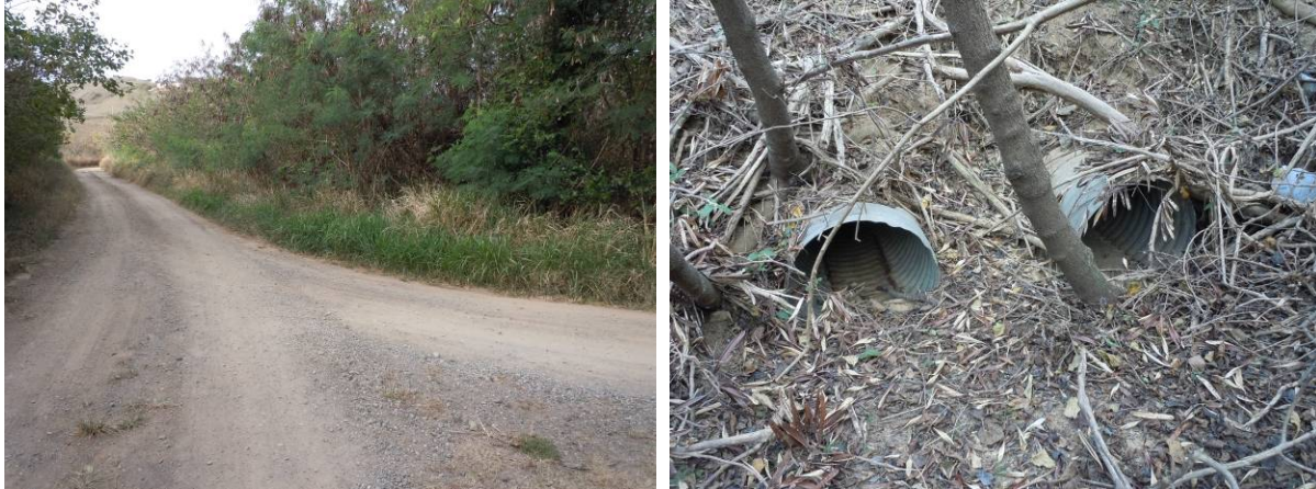
Figure 22. Portion of road that crosses the gut to the northeast (left), and the two 24-inch corrugated metal culverts at the gut crossing (right).
