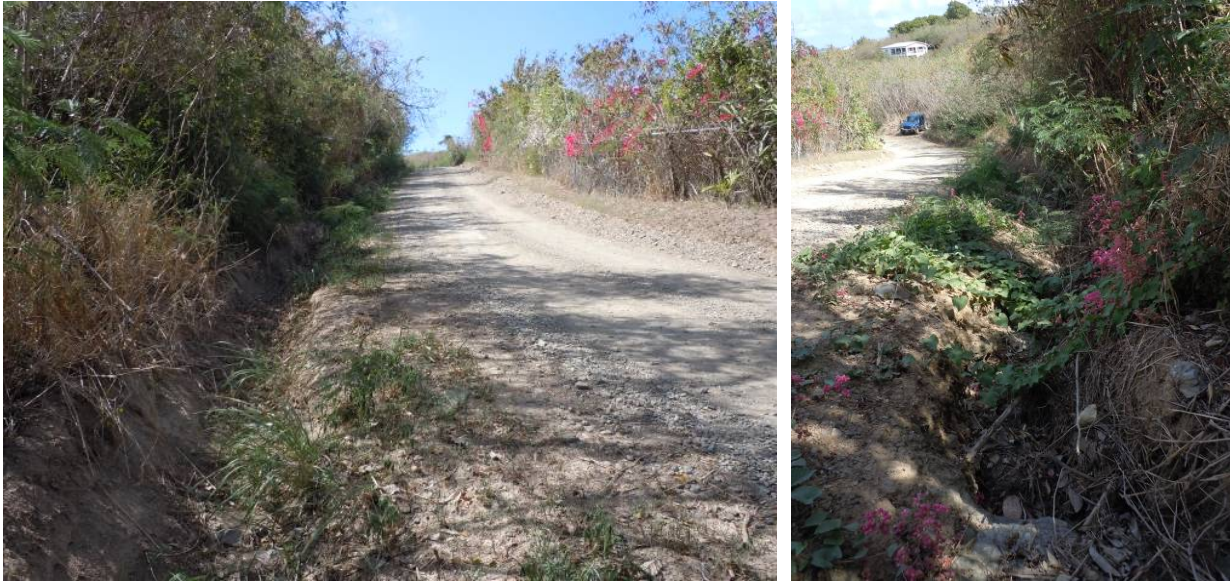
Figure 18. Looking uphill and downhill along the steep portion of this segment; the eroding ditch on the inslope is evident.
