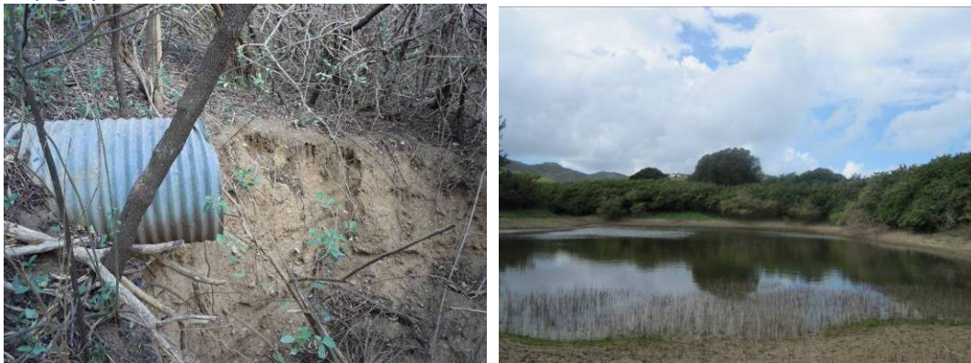
Figure 4. Large scour hole in the main gut, downstream of the 30-inch culvert under Pony Club Trail at entrance of Hope and Carton Hill (left). Further downstream, a large pond provides storage and habitat in the gut (right).
