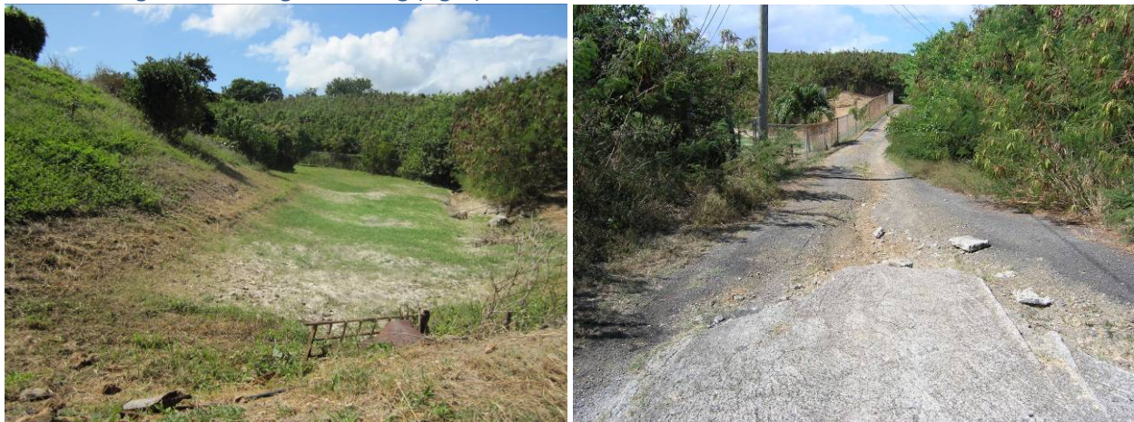
Figure 43. Gut downstream from large pond with two damaged/clogged culverts (left); the deteriorating road at the gut crossing (right).
