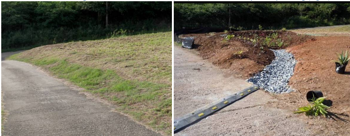
Figure 41. Before the rain garden was constructed (left) and immediately after planting (right).
