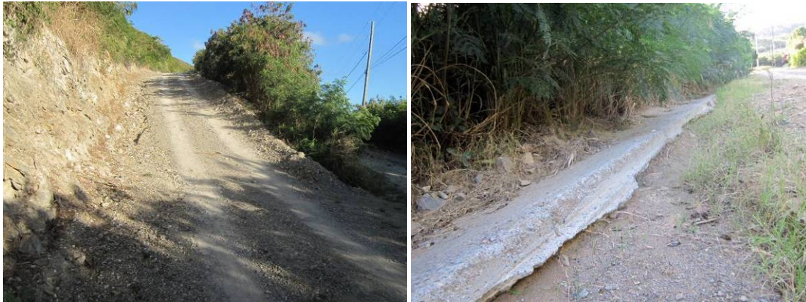
Figure 7. Roads in the Hope and Carton Hill Neighborhood are unpaved and very steep (left). Runoff from this road bypasses and undermines the paved swale (right).
