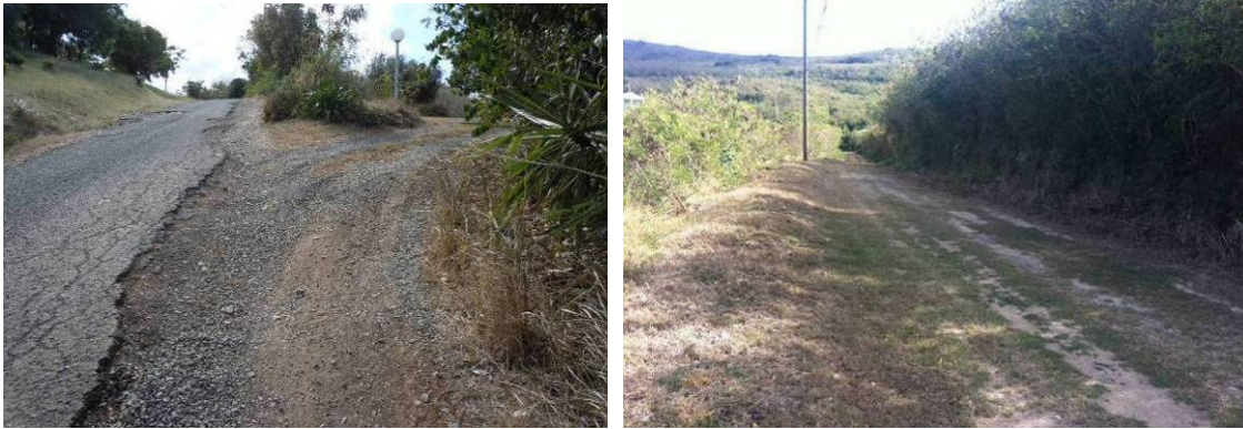
Figure 15. Broken asphalt along Divi-Divi Trail (left), and a grassy section of the road where the slope is flatter, little erosion has occurred, and some evidence of ponding was observed (right).
