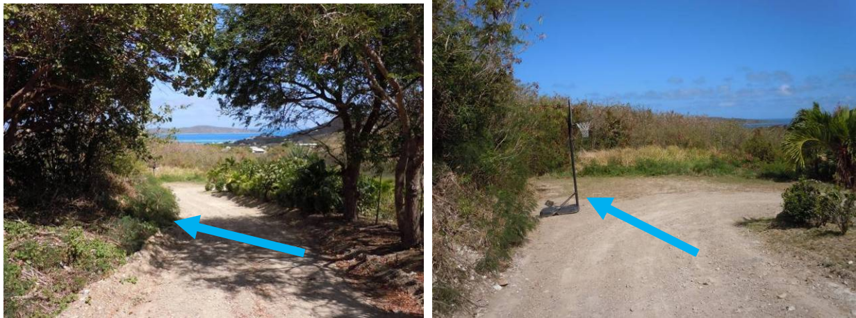
Figure 24. Runoff from the last portion of Ginger Thomas Trail flows to the western side of the road (left), towards the flat turnaround area where there were some signs of ponding (right).
