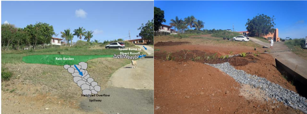
Figure 40. Initial rain garden concept (left) and finished rain garden (right), constructed as a part of a volunteer work day in October 2012.
