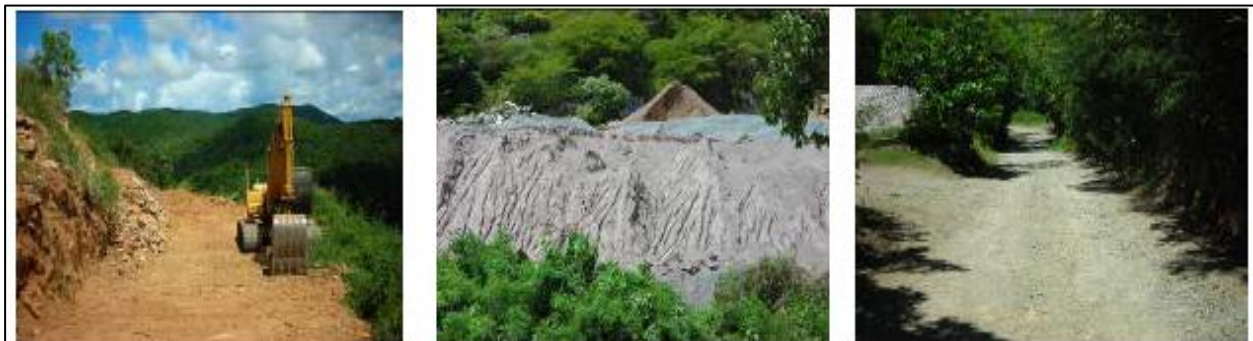
Photo 4: Sediment sources in Fish Bay including land clearing, construction materials storage, and unpaved roads.
