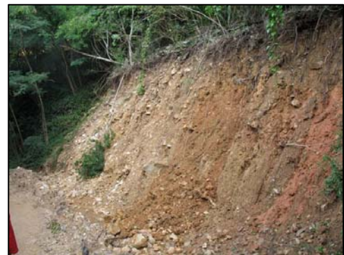
Photo 8: Road cut-slope needing stabilization.
