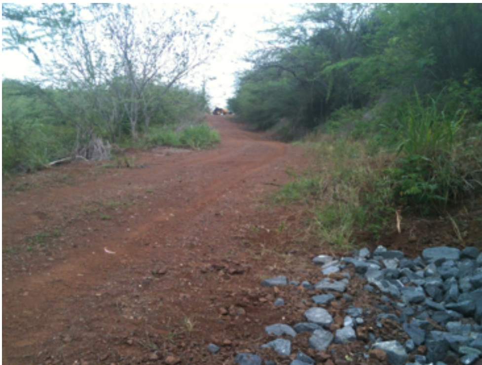
Figure 6. Note a series of check dams up the hill on the right (these slow the velocity of the water and drop out sediments) also the cross swale in Figure 3 was constructed midway up the hill to reduce the drainage area of the flowpath. The rocks in the foreground attenuate flows coming from the opposite direction.
