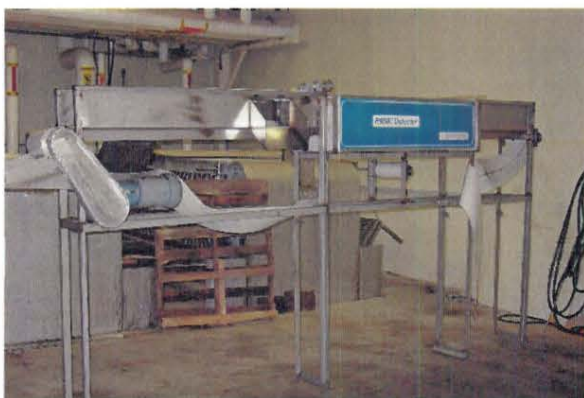
Detection unit conveyor line
