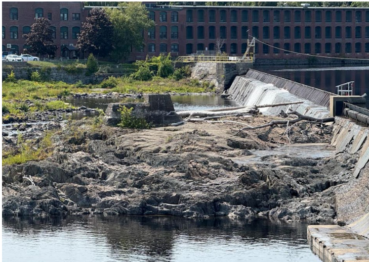
Figure 5. The approximate location of the proposed spillway diversion wall. The wall be constructed on top of the ledge just downstream of the dam.
