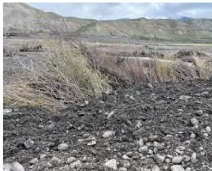
STAGE 3: TRENCH BACKFILLED WITH NATIVE ALLUVIUM AND ORGANIC TOP LAYER BEING PLACED.
