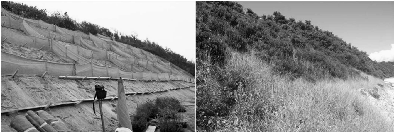
Figure 1. Erosion of a soft bluff can be mitigated by regrading the bank to a stable slope and then planting it with appropriate vegetation to provide a stabilizing root system. This project used a baffled cell technique and biodegradable matting to provide protection while the native plants became established. Temporary scaffolding was erected to reduce soil compaction and erosion during the construction phase. The mature native plants withstood Hurricanes Irene and Sandy with no major erosion, bank sloughing, or plant loss (New England Environmental, Inc., 2015; photo credit: New England Environmental, Inc.).
