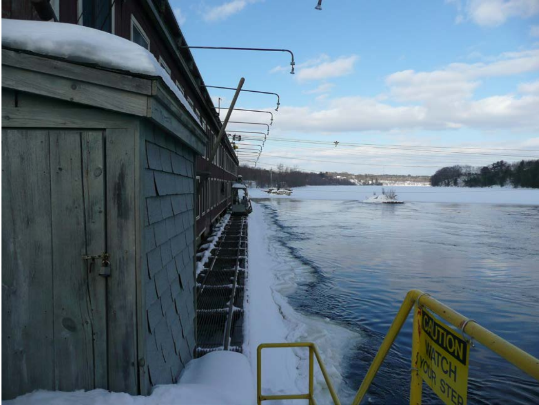
Figure 5. Veazie Project Powerhouse B and view of impoundment from west bank of the Penobscot River. (Source: Staff)
