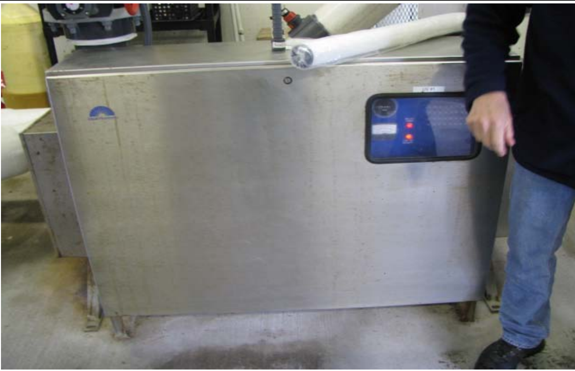
Photo 3: UV system used to treat filtered seawater that will go into the fish tanks.
