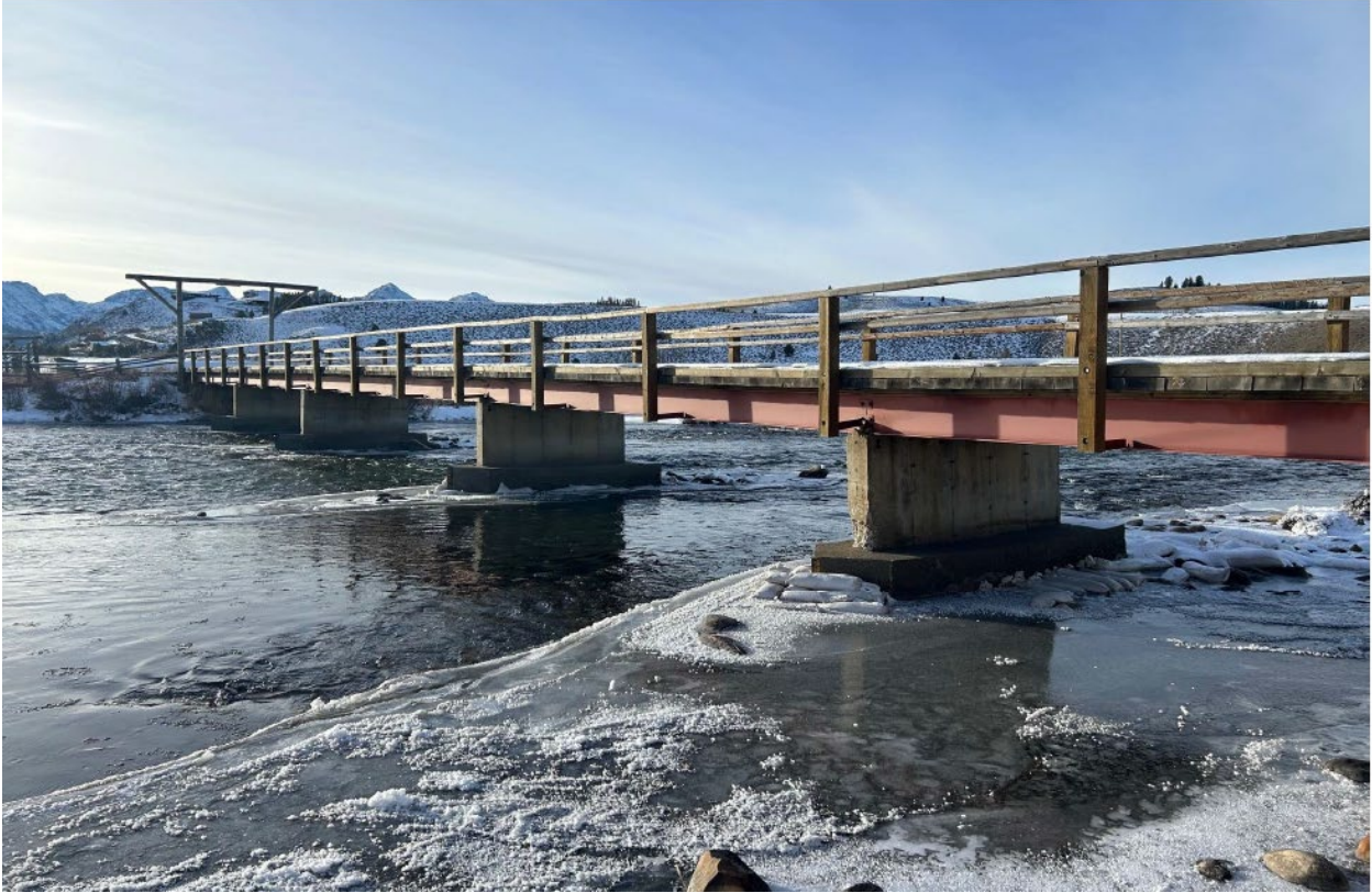
Figure 1. Cassidy Bridge and temporary sandbags placed on March 20, 2023, at the two eastern piers (foreground).
