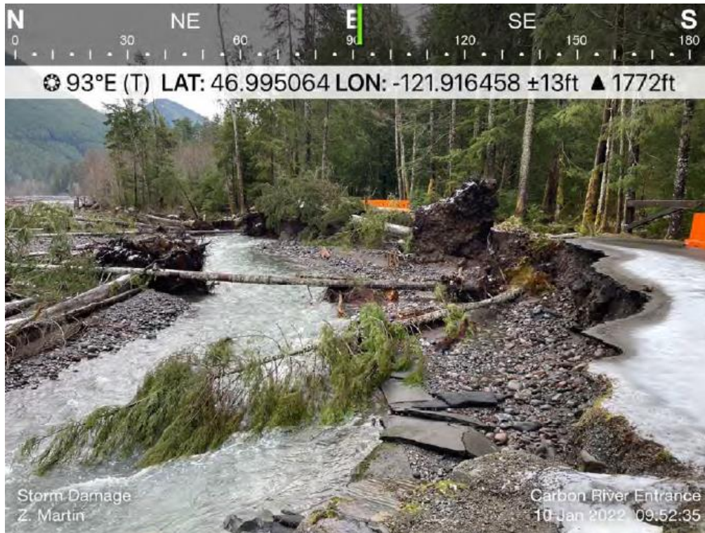
Figure 1. Carbon River Road segment following high flows in January, 2022.
