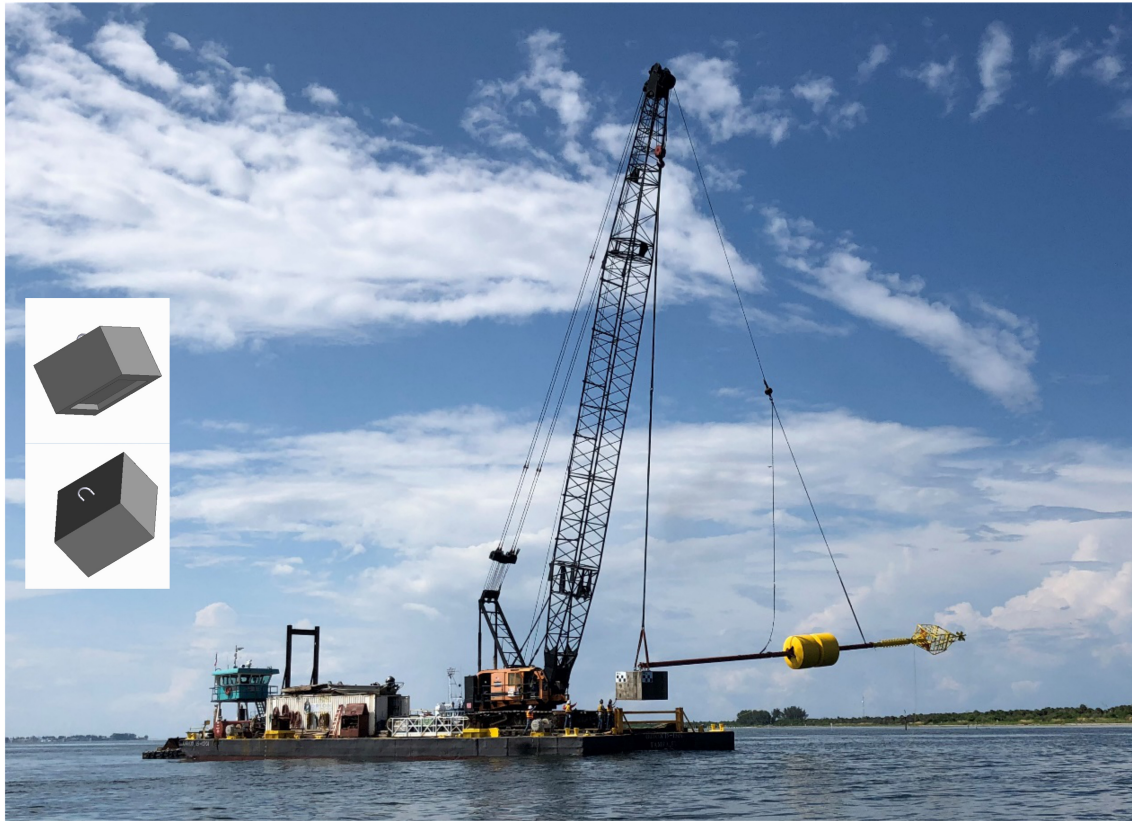
Figure 3. Deployment of assembled mooring. Main winch line is attached to the anchor, while the auxiliary line with two-point sling supports the spar section. Inserts show design of the ballast, note indented bottom.
