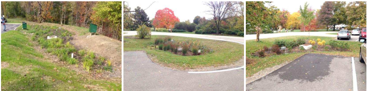
Figure 3. The UC (left) bioretention cell six months post-construction and the HA South (middle) and North (right) bioretention cells 13 months post-construction.
