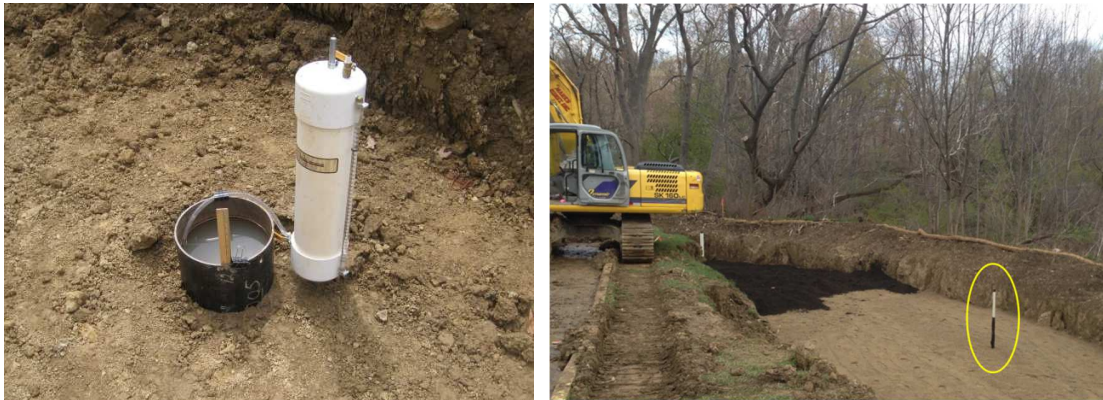
Figure 4. Single ring infiltrometer with Mariotte bottle used for pre-construction infiltration testing (left) and monitoring well used for post-construction drawdown rate measurement (right).
