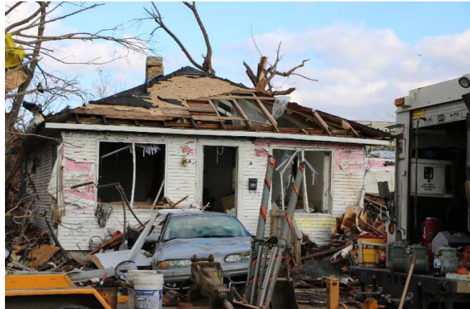
Fig. 4. DOD 4 building in Naplate, IL with post-storm structural functionality of SF 0.1.
