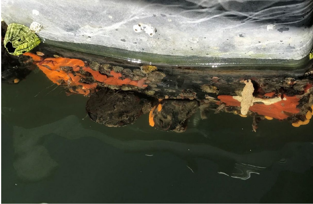
Figure 3. Photo of encrusting organisms on a floating dock to be removed during the Project (Moffatt and Nichol 2022).
