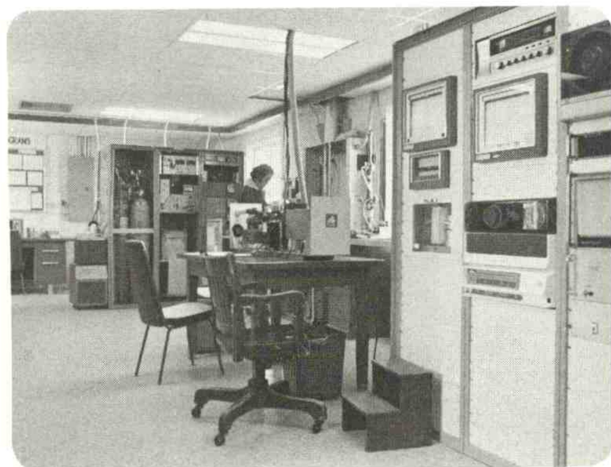
In 1978, in the newly modernized main building, Alan Yoshinaga is checking air inflow from the air sampling intake stack.
