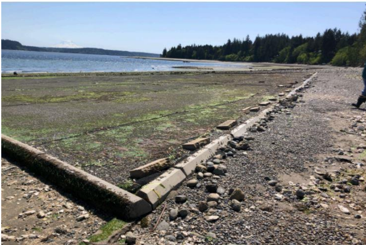
Figure 2. Image of curbs and anti-predator netting previously installed
