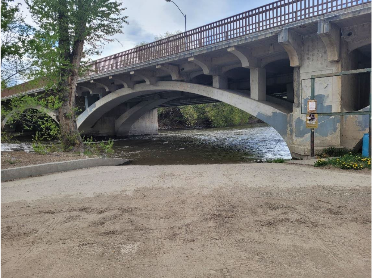
Figure 2. Existing concrete boat ramp immediately upstream of U.S. Highway 93 Bridge on west channel of Salmon River. Lower segment of ramp will be cut off, replaced, and then extended by 10 feet in length.
