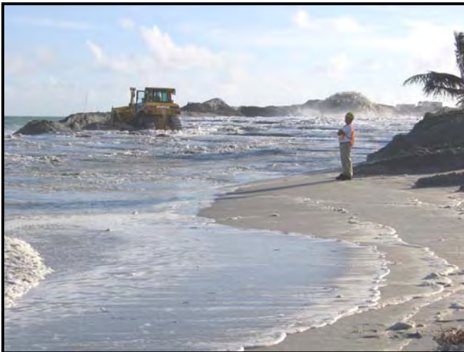
Sand Dike being constructed during slurry discharge at John U. Lloyd Park in Broward County, FL. Source: FDEP
