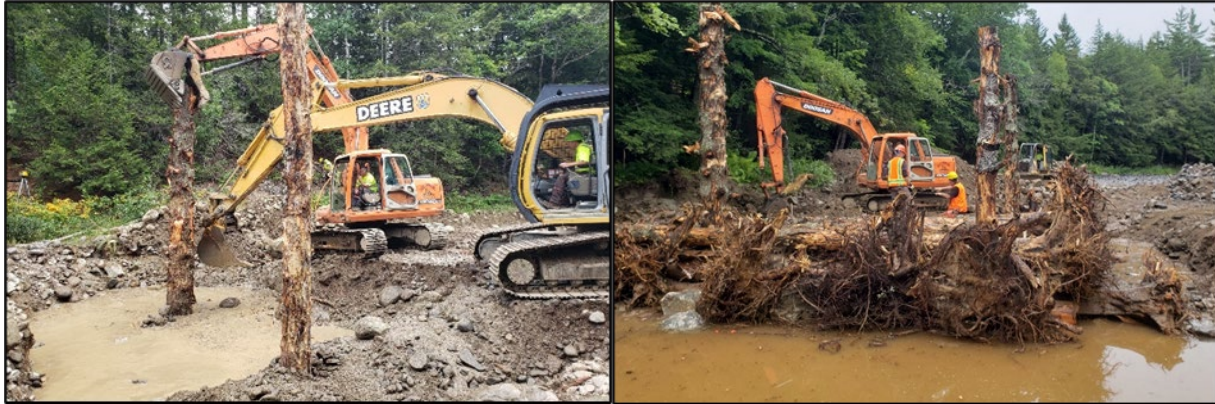
Figure 3.3.2. Photos of the installation of engineered log jams into the Narraguagus River Restoration Project at Rt 9 Pilot site.
