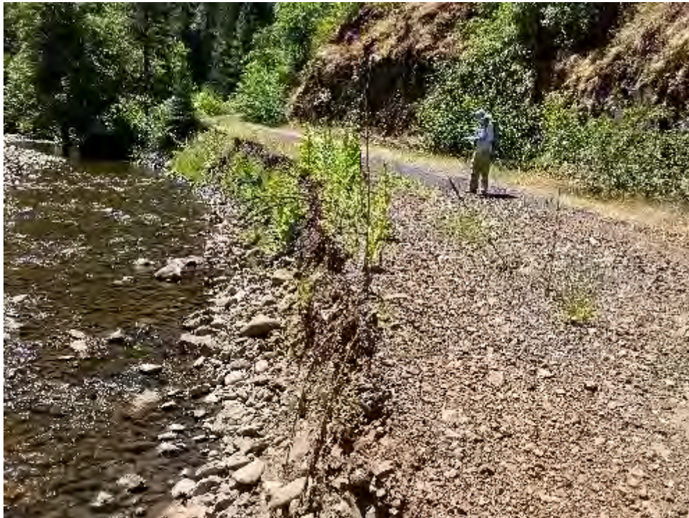
Figure 1-5: Road and bank erosion at MP 1.52, looking upstream
