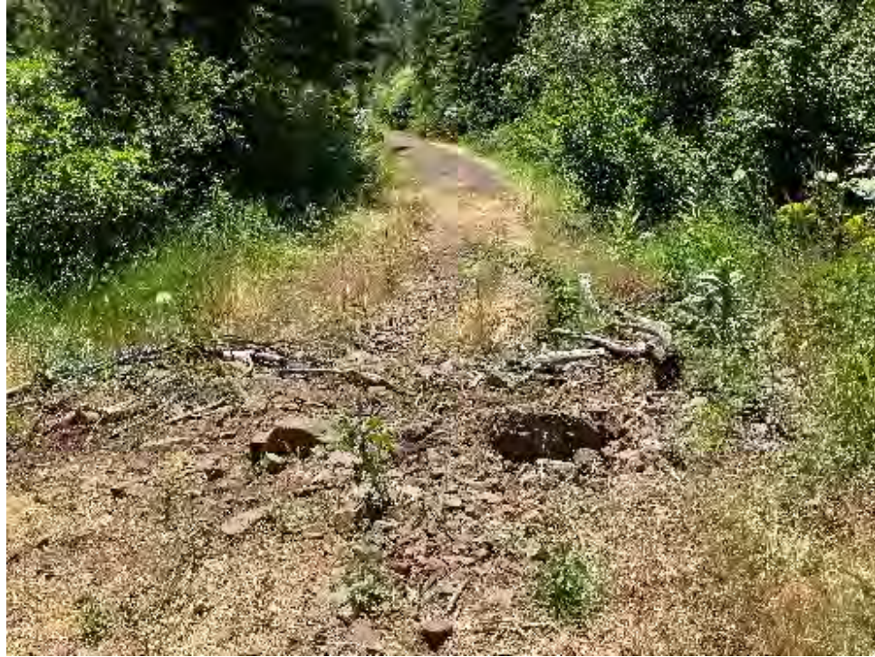
Figure 1-15: Debris slide at MP 1.26
