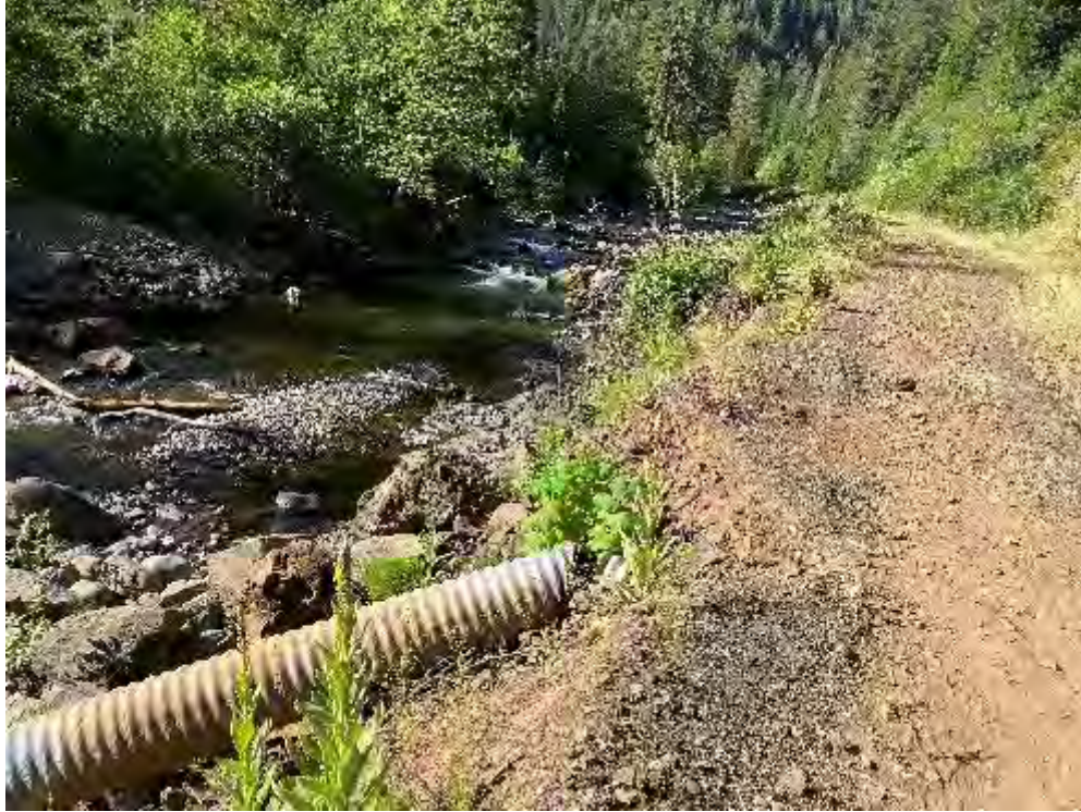
Figure 1-2: Culvert and bank damage at MP 1.30
