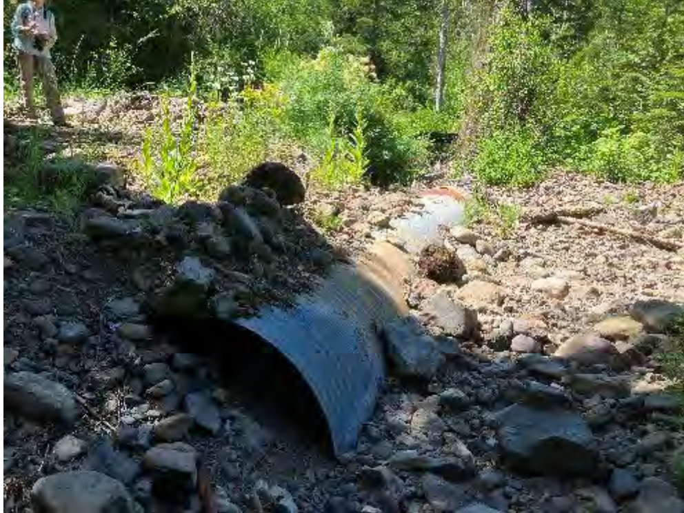
Figure 1-9: Washed out culvert at MP 2.54
