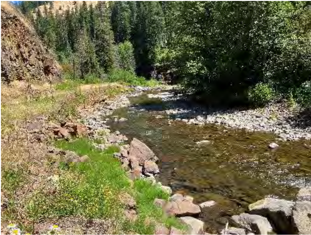
Figure 1-4: Road and bank erosion at MP 1.38, looking downstream
