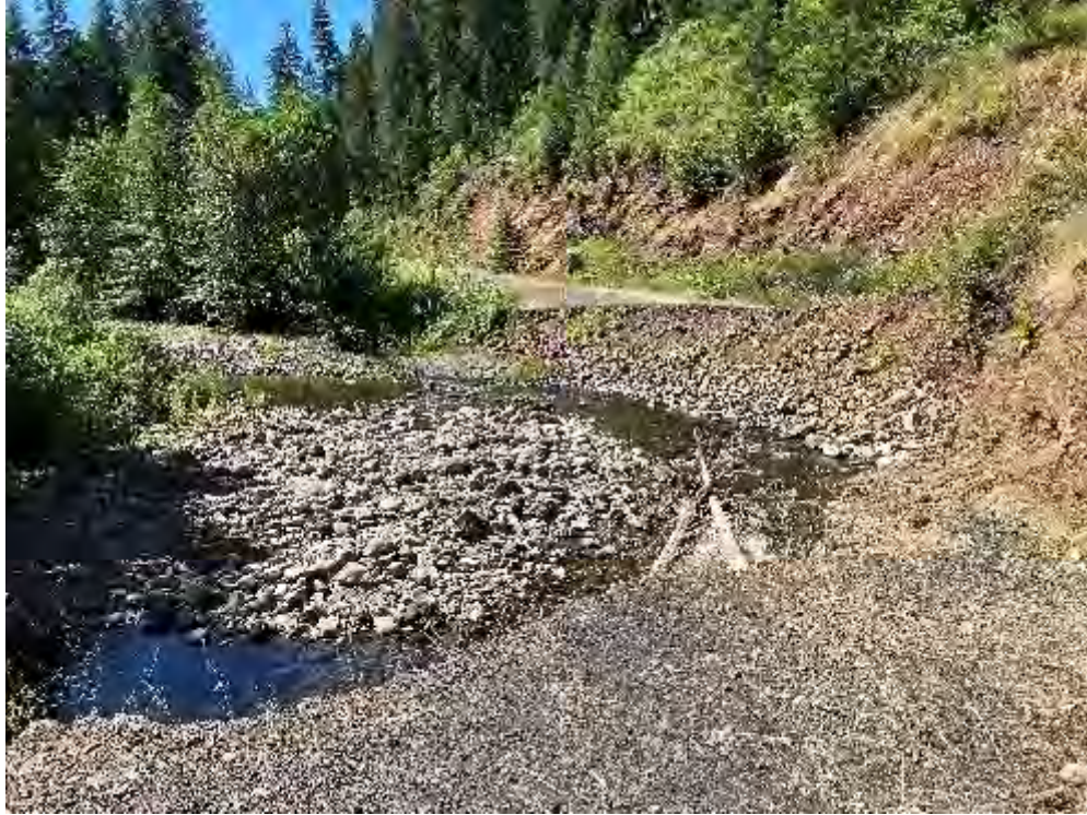
Figure 1-3: Road washout at MP 3.08, looking upstream
