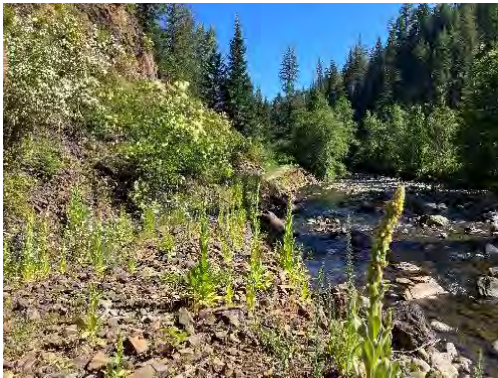
Figure 1-53: Washout at MP 3.53, looking downstream
