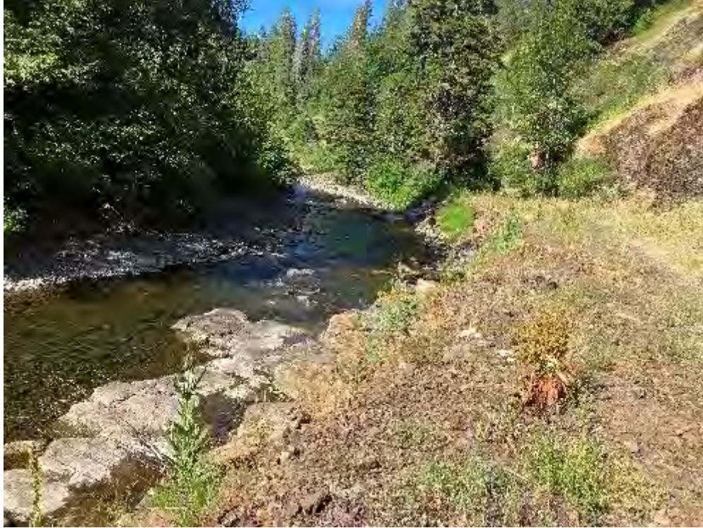
Figure 1-3: Road and bank erosion at MP 1.38, looking upstream
