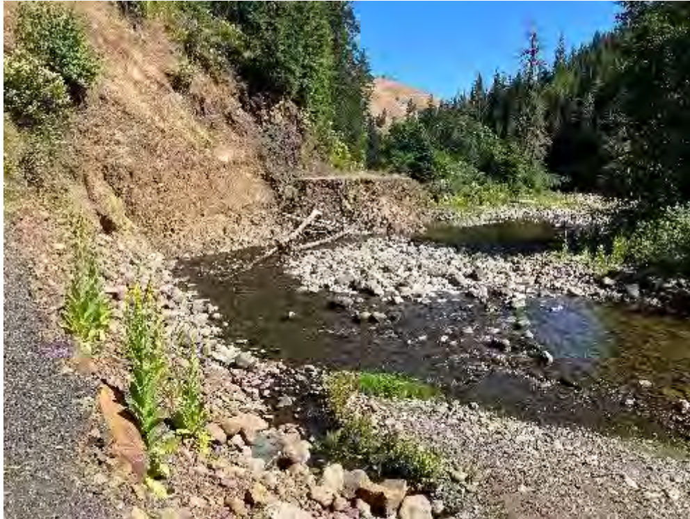
Figure 1-20: Road washout at MP 3.08, looking downstream
