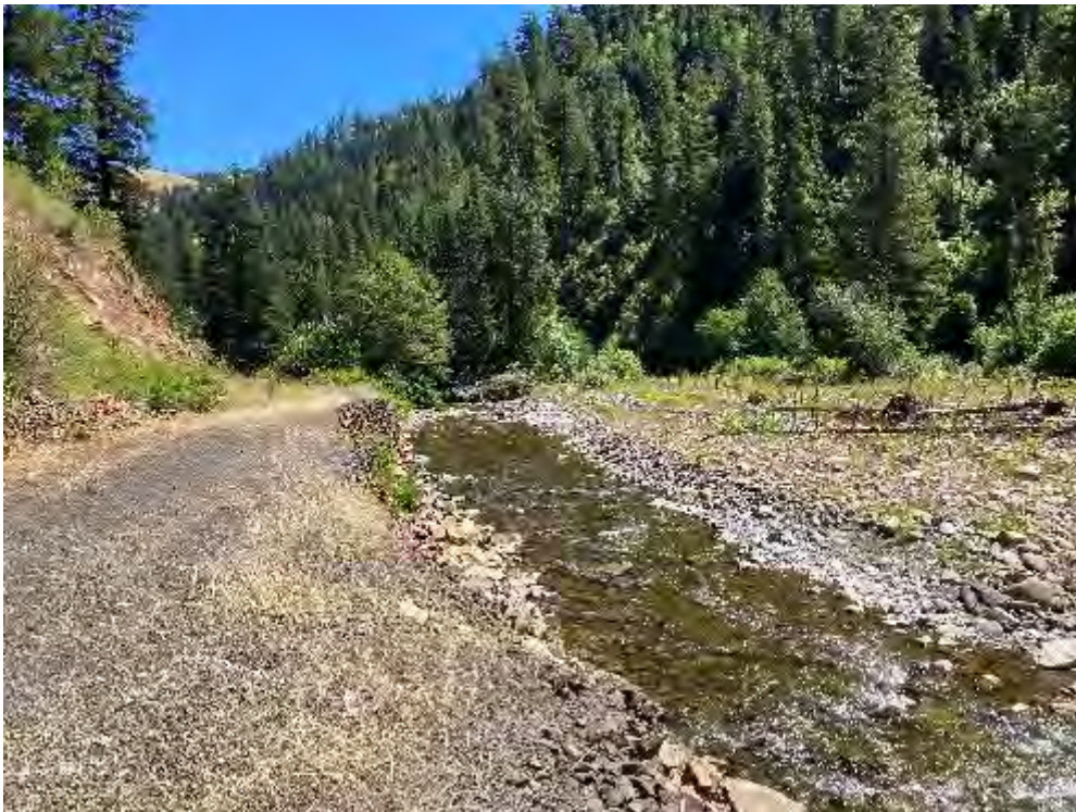
Figure 1-6: Bank erosion at MP 1.96, looking downstream
