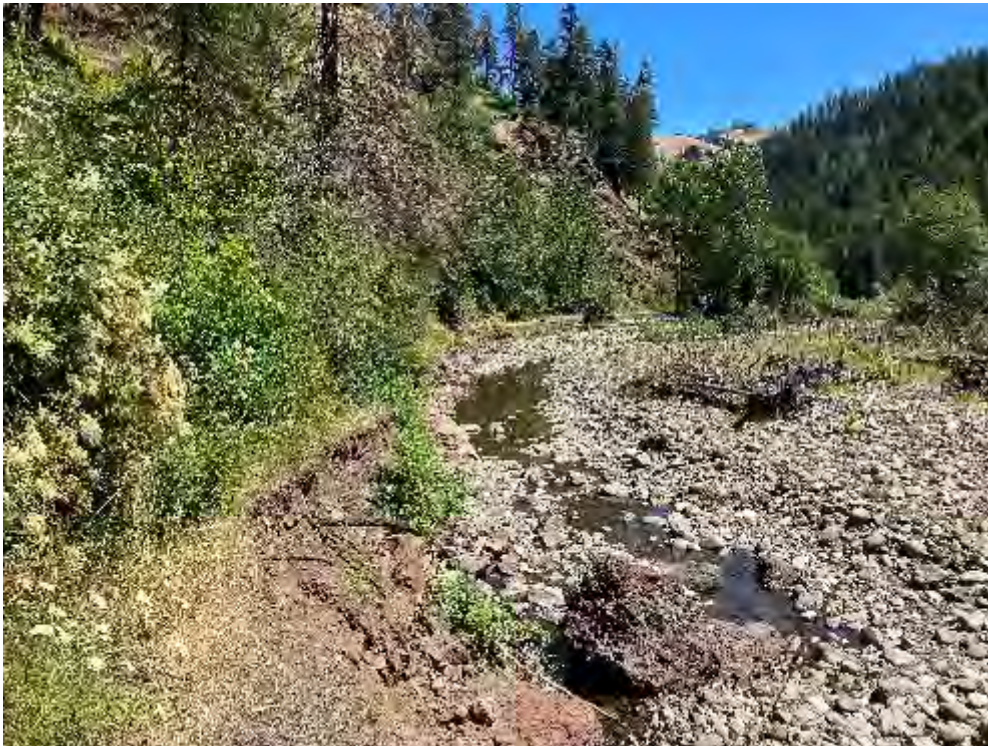
Figure 1-7: Road washout at 2.02, looking downstream
