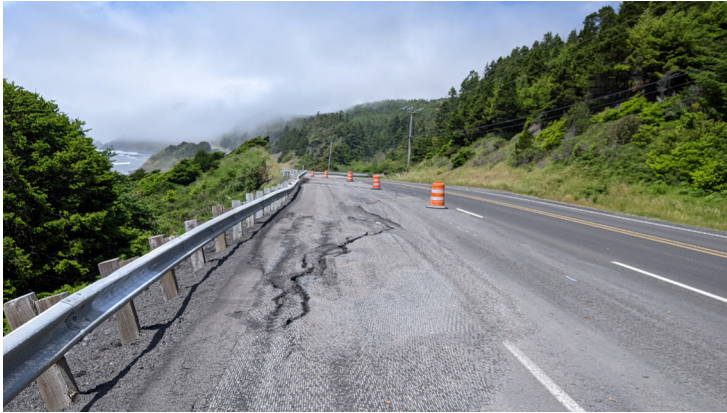
Figure B1. Damage resulting from a landslide along an unstable, erosion-prone section of U.S. Highway 101 south of Port Orford, Oregon (June 2022). Photograph by Michael Olsen.
