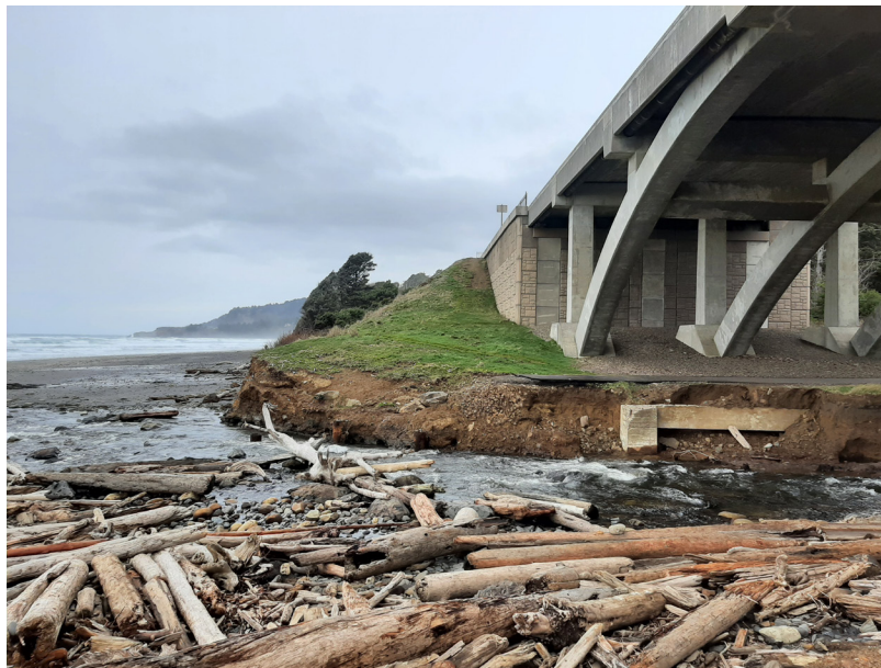
Figure 4. Coastal erosion at Beverly Beach and U.S. Highway 101, Lincoln County, Oregon, February 2021. Photograph by Hailey Bond.
