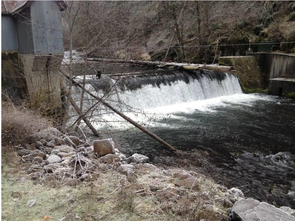
Photo 1. CWWID looking upstream from north bank to dam crest. November 2012 – flow is about 150cfs, over 100cfs greater than flows anticipated during summer debris removal activity.
