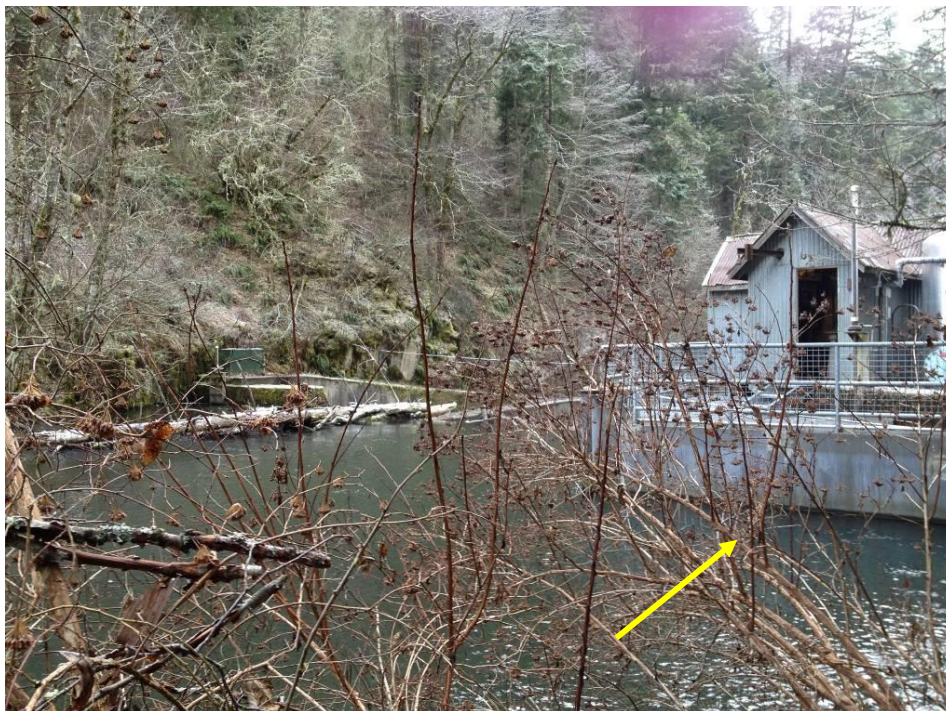
Photo 5. View of intake building on north bank. Bypass would convey flow through opening at base of concrete guide wall, and through sluice gates on face of dam, as shown by arrow.
