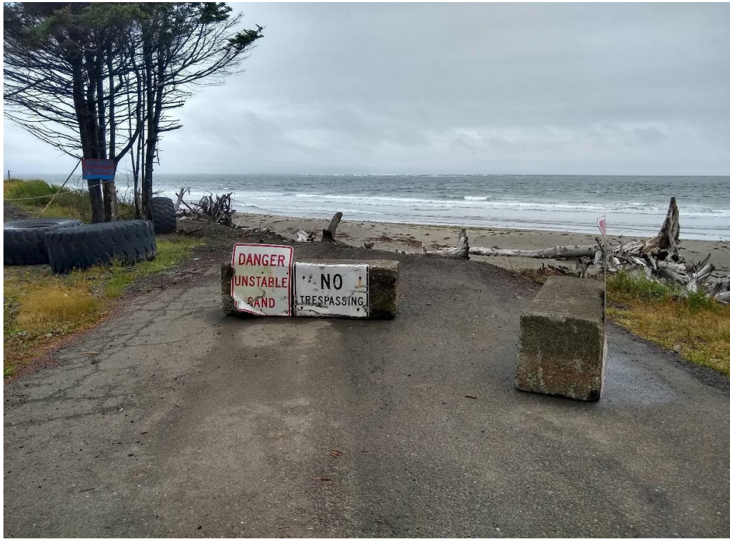
Figure 2. an eroded road ends abruptly on the beach in North Cove, Washington. July 2019 photo by Ian Miller, Washington Sea Grant
