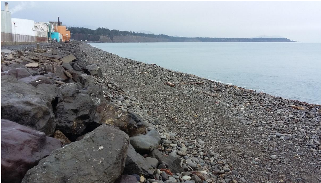
Figure 6. Cobble nourishment on Ediz Hook, Washington is placed approximately every 5 years to protect larger rip-rap material from undercutting. February 2017 photo by Ian Miller, Washington Sea Grant.
