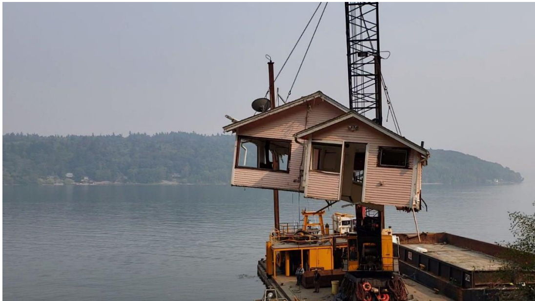
Figure 4. A home being removed from the shoreline in King County, as part of an ecosystem restoration project. Photo by Greg Rabourn, King County.
