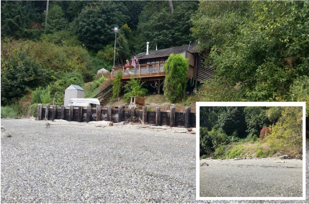
Figure 16. Before and after (inset photo) of a shoreline property on Vashon Island purchased by King County for a shoreline restoration project. Both the home, and the shoreline armor were removed in this project. Photos by Kollin Higgins and Greg Rabourn, King County.
