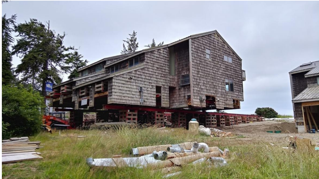
Figure 15. Multifamily housing moved back from a bluff due to erosion on Whidbey Island in 2018. Source: DB Davis Structural Moving and Raising, Island County, Washington. Reproduced with permission.
