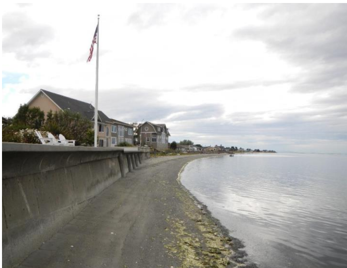
Figure 3. Extensive armoring along the shoreline near Sequim, Washington. August 2013 photo by Ian Miller, Washington Sea Grant.
