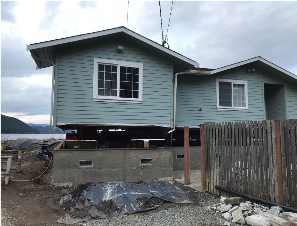
Figure 13. Examples of a home on Guemes Island undergoing elevation retrofits due to flooding. Source: DB Davis Structural Moving and Raising, Island County, Washington. Reproduced with permission.
