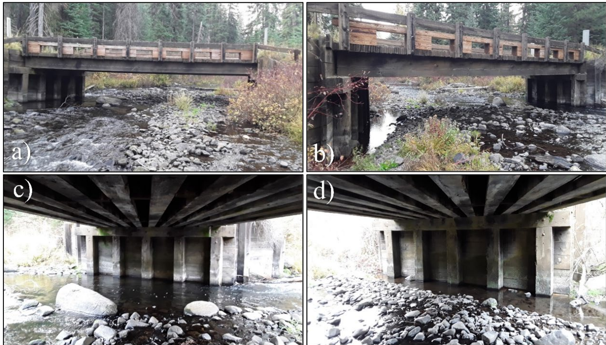
Figure 2. Photos of Boulder Creek Bridge 50074-17.88 with views of the: (a) downstream side of the bridge; (b) upstream side of the bridge; (c) east abutment; and (d) west abutment.
