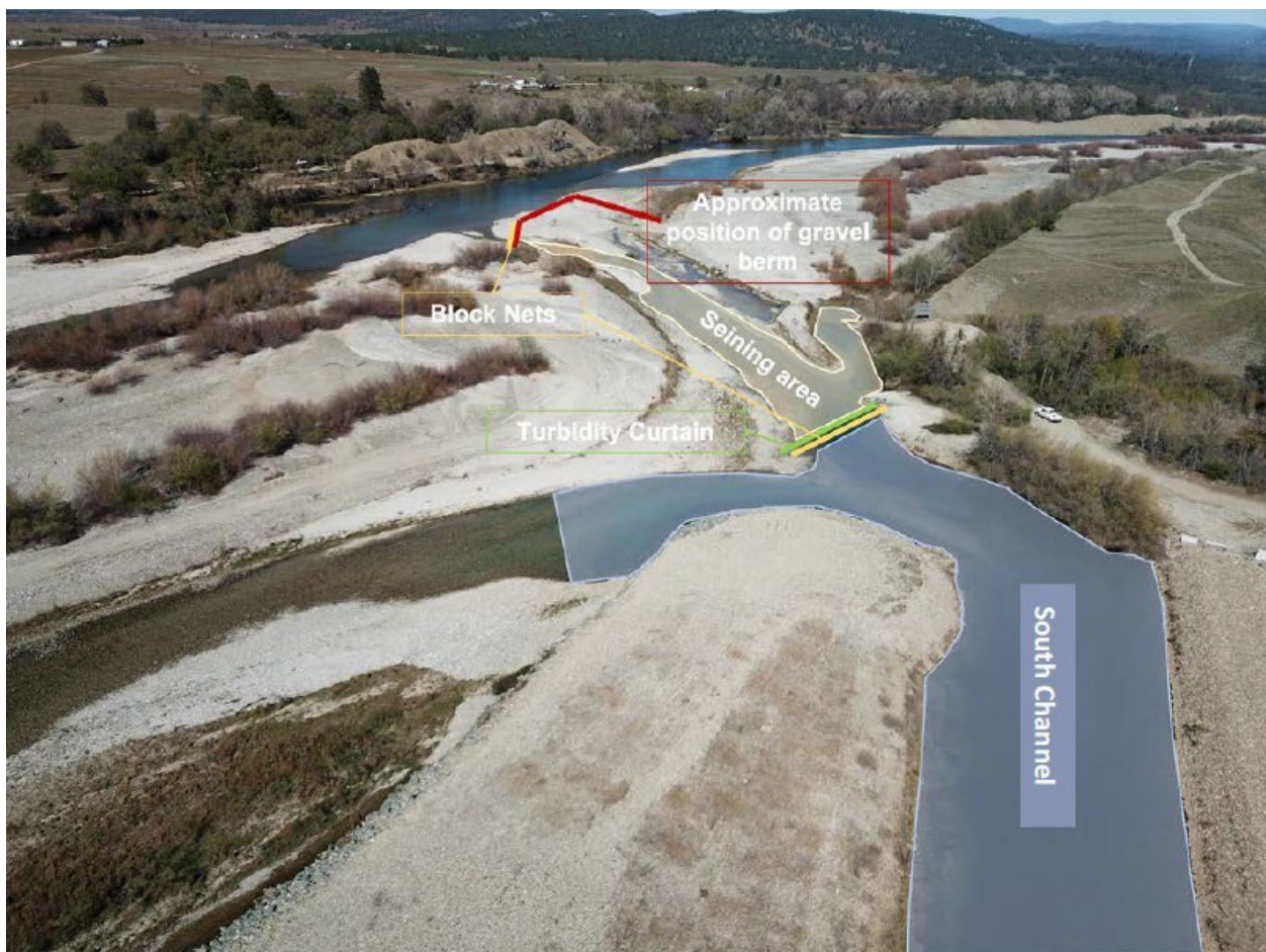
Figure 1. Example of where fish avoidance measures were used in 2022 prior to excavations.
