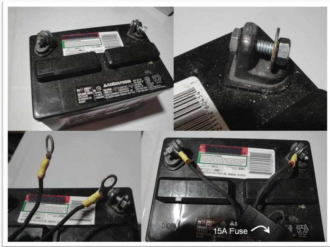
Figure 6-33. External 12V lawn mower-type lead-acid battery, with connectors to power a GNSS receiver.
