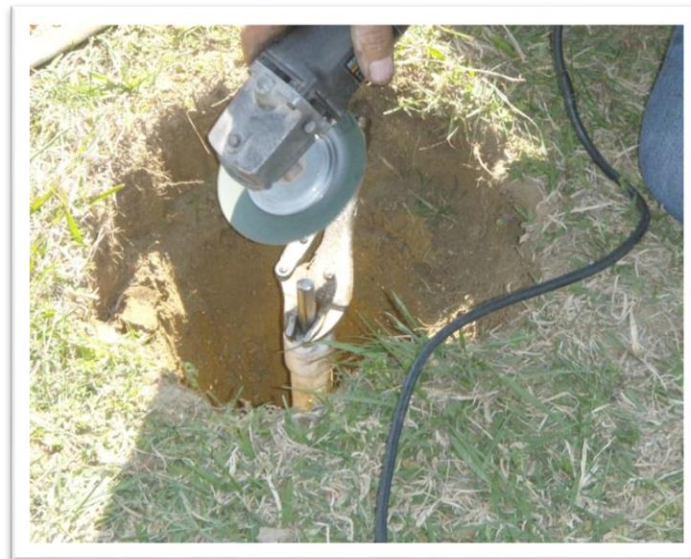
Figure 5-6. Using a cordless angle grinder to create a dome at the top of the rod.
