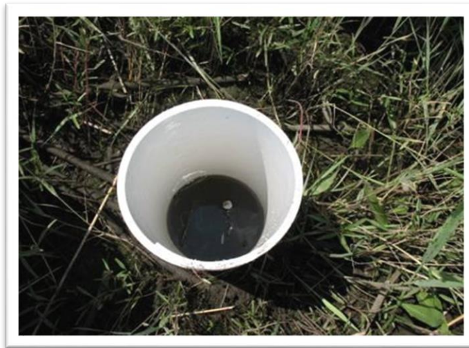
Figure 5-7. Inserting 15 cm PVC pipe in hole after section rods have been driven.
