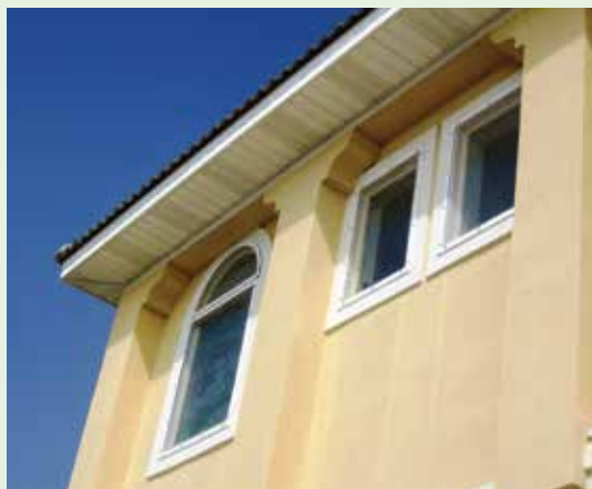
Figure 5-16. Flat impact polycarbonate panels are installed directly over windows of a coastal home. This window covering provides excellent storm protection with minimal aesthetic impact. Image courtesy of Roll-a-way
