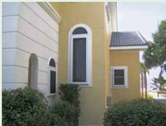
Figure 5-15. In-place stainless steel impact screen protects several windows of a coastal residence. This system requires no deployment and provides shade. Image courtesy of Roll-a-way
