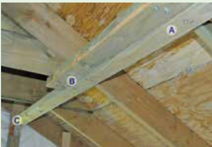
Figure 5-3. In this application of lateral bracing, the 2"x4"s are 18 inches from the ridge and connect to horizontal members that attach the opposing trusses. Not all roofs will have the horizontal members. The 2"x4"s are connected with two #14 3-inch screws (A) and overlap over two trusses (A and B). The end is connected to the gable end with an angle or L bracket (C). Image courtesy of Dennis Hwang
