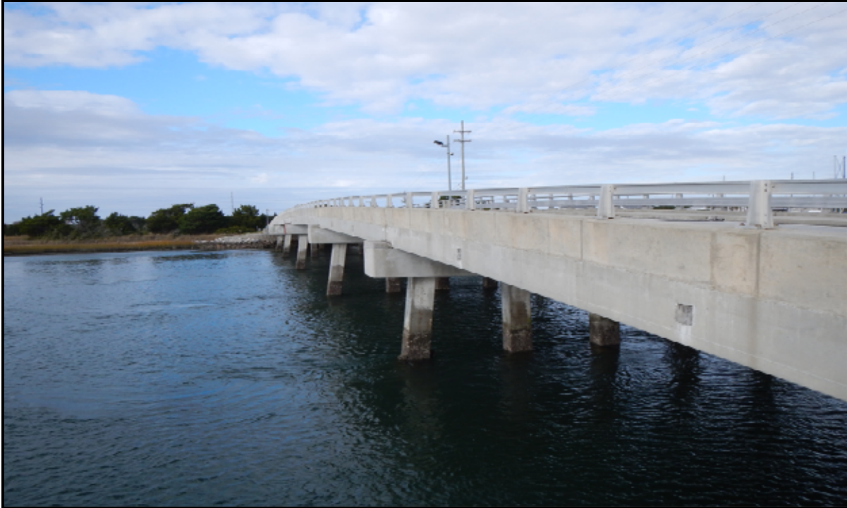
Photograph 5: View of the northern access bridge from the southern headwall facing north.
