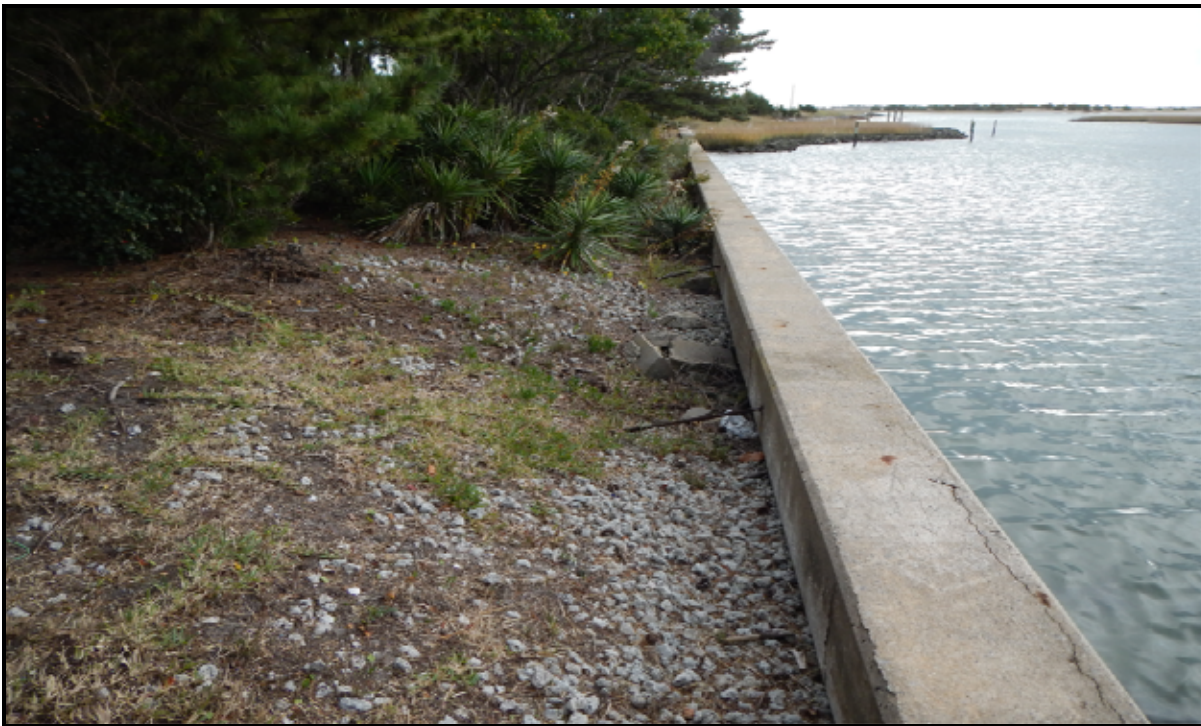
Photograph 12: Example of settling behind existing seawall that is causing the structure to fail and present erosion hazards on the western shore of Pivers Island.
