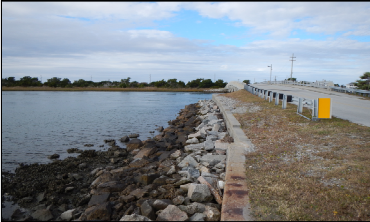
Photograph 4: View of the seawall adjacent to the northern access bridge facing north.
