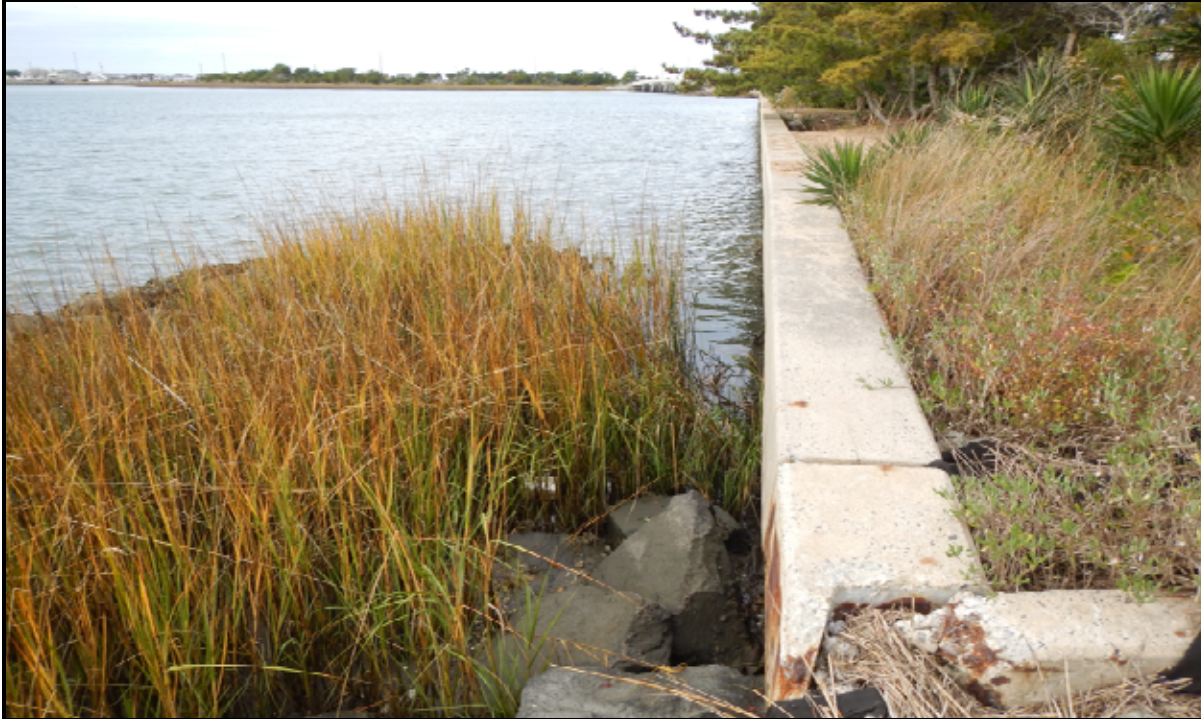
Photograph 2: View of the seawall at the southern limit near the Duke University property facing north.
