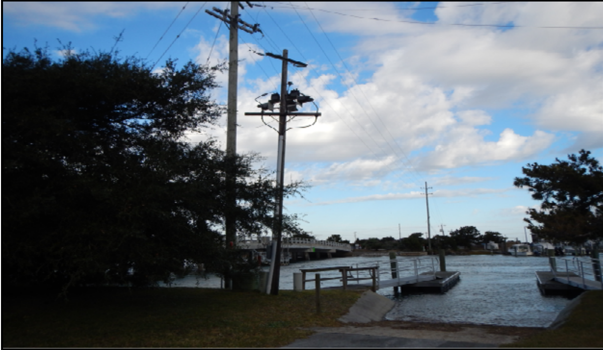
Photograph 1: Aerial crossing of electrical service o the CCFHR campus and Duke University. The pole with the down conduit is the split off of Duke University’s electrical service.
