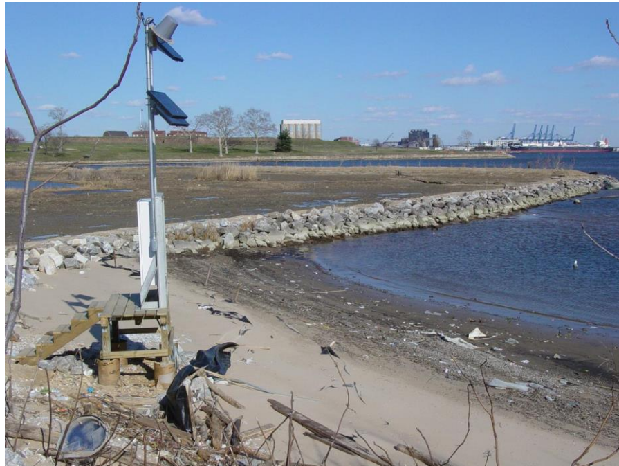
Figure 12. The 1-year tide station at Ft. McHenry Marsh with the equipment shelter and Geostationary Operational Environmental Satellites (GOES) antenna and solar panel towers.
