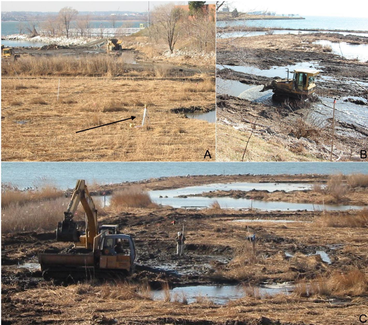
Figure 11. (a). The use of the leveling transit to control the wetland surface. (b). The grading of the surface of the wetlands. (c). The use of leveling rods to determine the depth of one of the ponds being sculpted by the heavy machinery.
