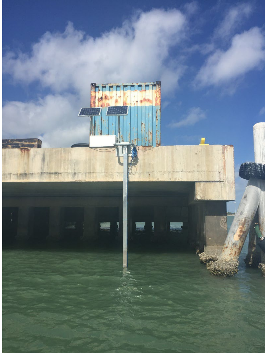
Figure 3-4. I-Beam attached to a pier with solar panels and white electronics enclosure box.
