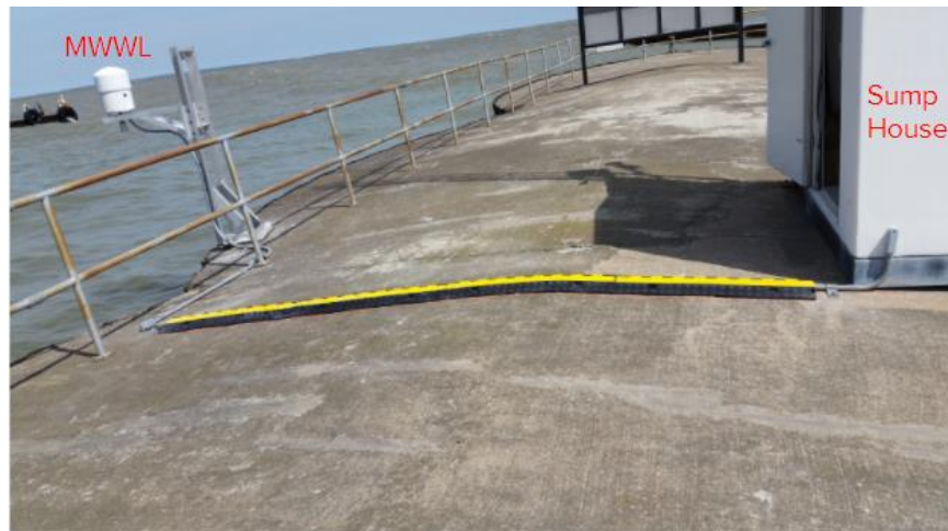
Figure 20. Locations of the sump house where the primary National Water Level Observation Network (NWLON) station is located and the microwave water level (MWWL) station at Marblehead, OH.
