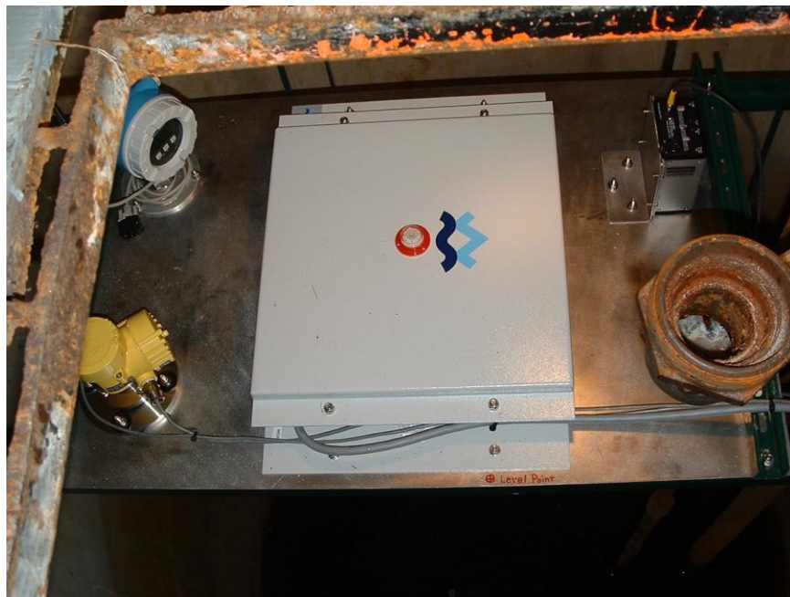
Figure 6. Fort Gratiot, MI, Microwave Water Level (MWWL) installation inside sump.
