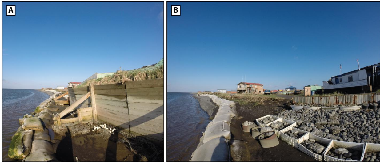
Figure 24. Seawall and sediment containers in place along the lagoon coastline of the community . A) the seawall and gabions, the geotextile containers can be seen on the left, and B) the geotextile containers fronting the community to the west of the seawall. May 2019.
