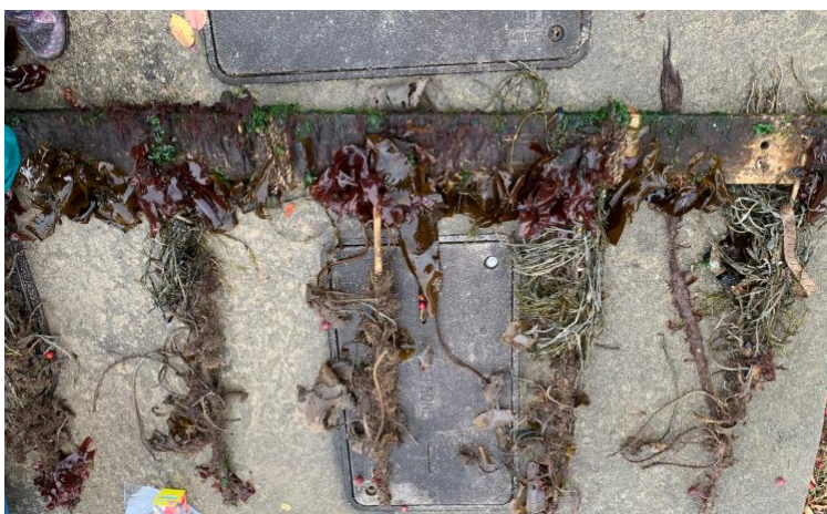
Figure 7: Image of biofouling accumulated on the composite line test structure
