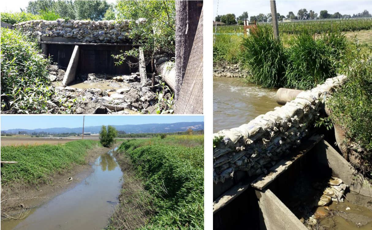
Figure 5. The existing weir at College Lake (top and right) and the primary ditch within the center of the lakebed upstream of the weir (bottom left). Source: Joel Casagrande, NMFS, June 2017.
