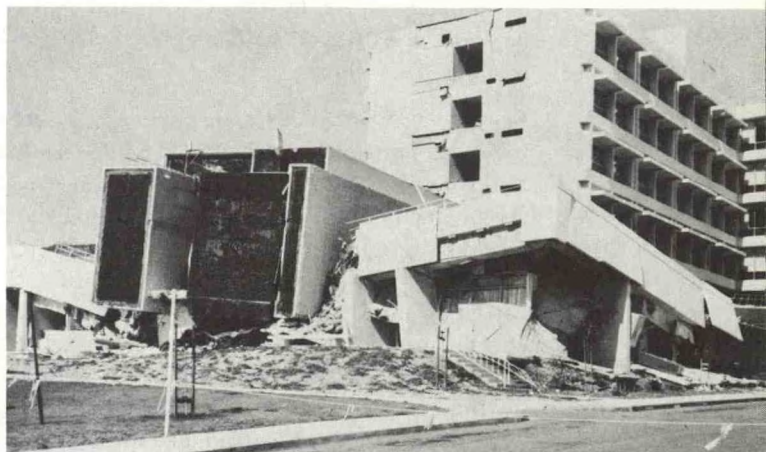
Overturned elevator and stair tower at Olive View Hospital.
