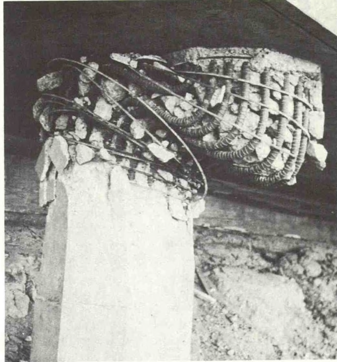
Distortion in supporting column of freeway overpass.
