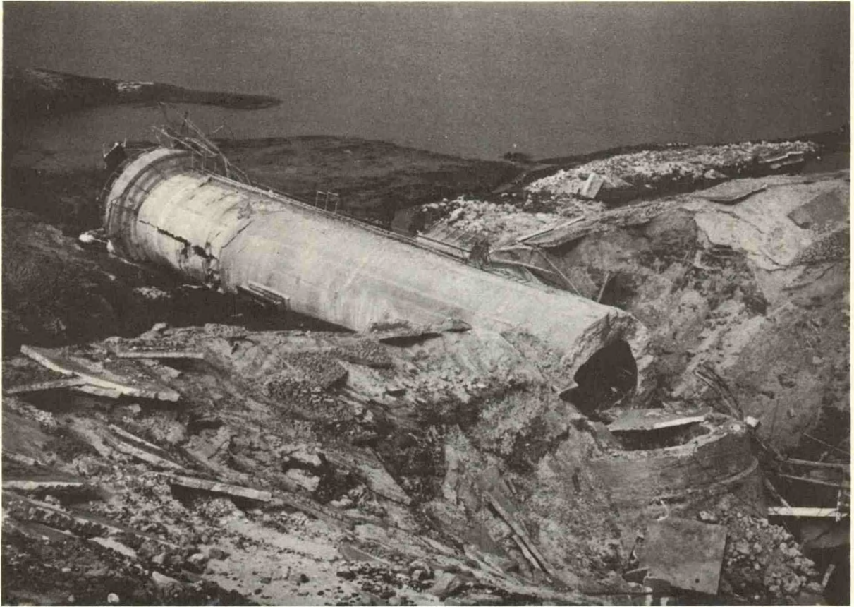
Van Norman Lake drainage tower snapped at base.
