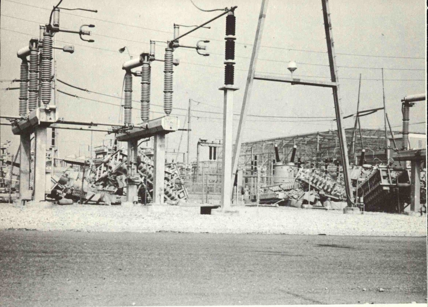
Damage at Sylmar Converter Station.
