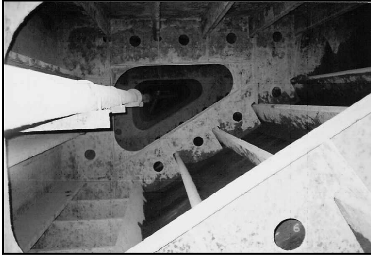
Figure 1-1: View inside an upper wing ballast tank. There are many structural components that provide traps for sediment and that may create dead zone during ballast water pump-out. Photo credit: Great Lakes NOBOB Program
