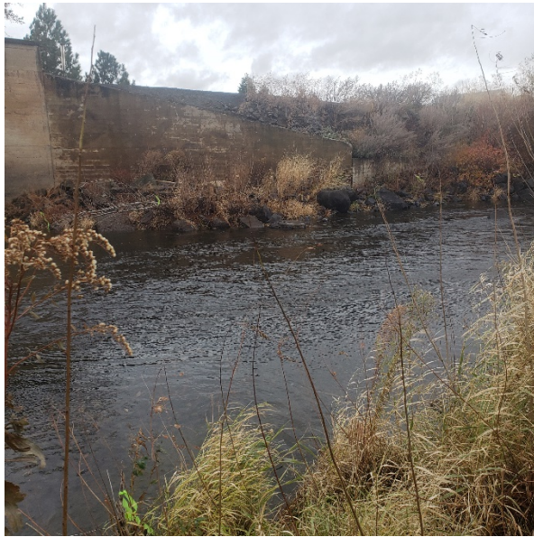
Photo 5. Bank armoring river right upstream of bridge.
