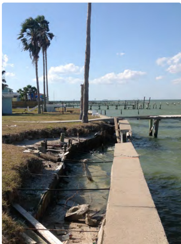
Bulkhead failure leads to erosion and land loss. Photo: Texas General Land Office
