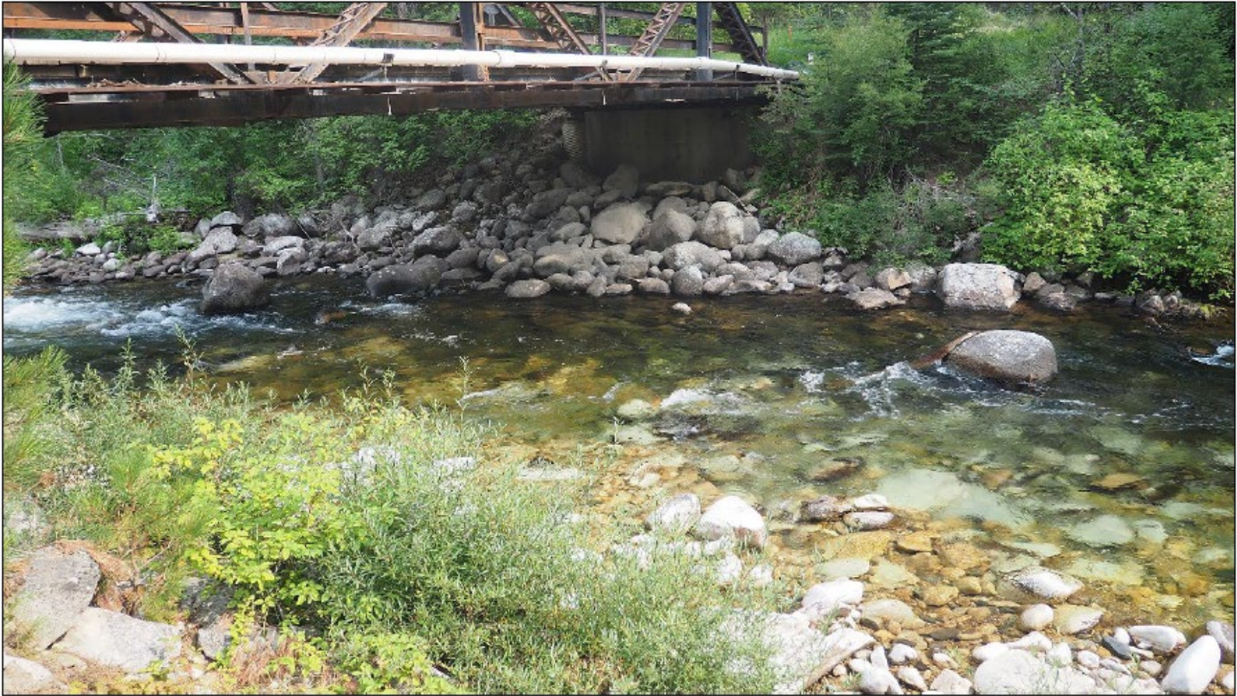
Figure A-2 View of aquatic and riparian habitat beneath the existing Abstein Road Bridge. The proposed locations of the abutments for the new bridge are at the bottom left and top right of the picture.
