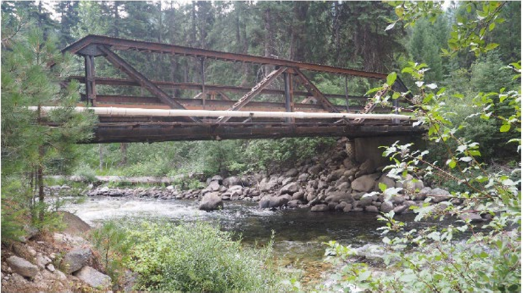
Figure A-1 The current Abstein Road Bridge from the north bank looking upstream.
