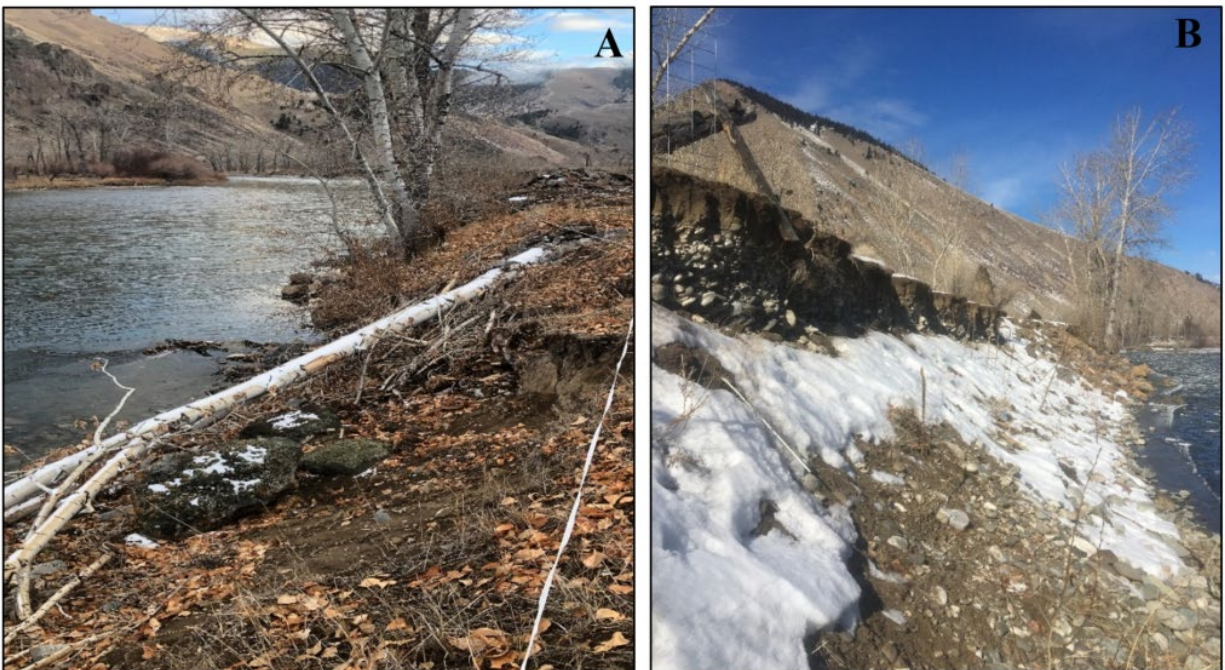
Figure 2. Photographs of the existing bank conditions. Photo A is a downstream view of the eroding bank above the segment armored in 2021. Photo B is an upstream view of the lower segment, below the recently completed bank armoring Conservation Measures.
