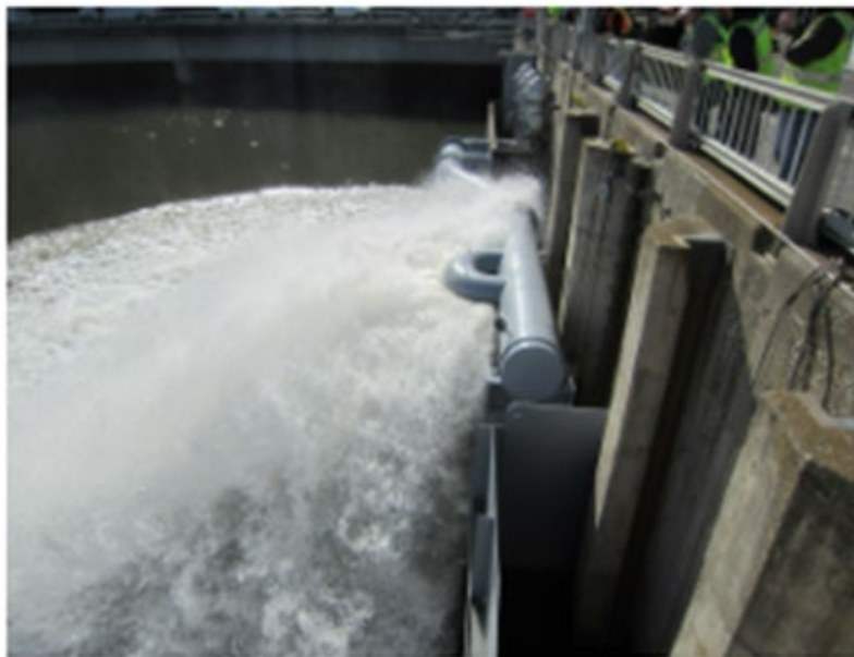
Figure 14 Spray System to Supply Cooler Water to the Adult Fishway at Lower Granite Dam, Washington
