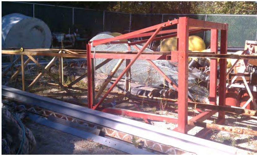
Figure 2: Corrosion on old turbine test structure
