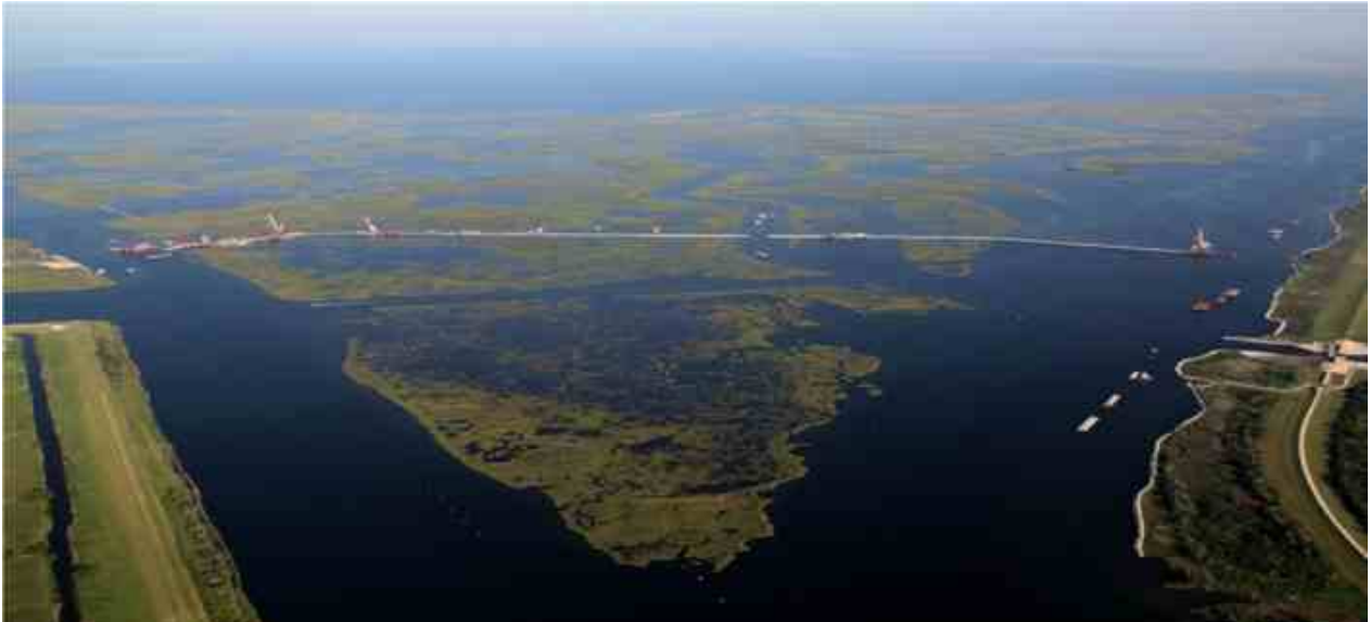
Figure 1. Top: Construction of the Inner Harbor Navigational Canal Surge Barrier (IHNC SB) across the Golden Triangle marsh near Chalmette, Louisiana. The remnant interior marsh is in the foreground (westward of the wall) and larger marsh is in the background (eastward of the wall). Image borrowed from the Internet without permission. Bottom: Study area with approximate locations of throw trap sample sites interior (red dots) and exterior (yellow dots) of the IHNC SB (blue line).
