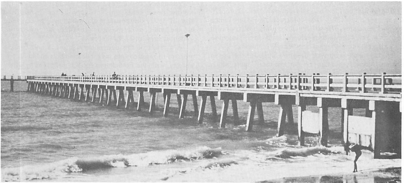
Reinforced concrete, when exposed to sea water, is subject to corrosion of the reinforcing metal and subsequent cracking of the concrete. The objective of this study has been to determine ways to minimize cracking and corrosion of such structures.
